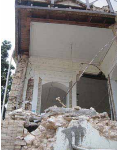
FIGURE 102 In this case the horizontal metal ties failed to prevent the collapse of these masonry walls, but may have helped prevent the collapse of the rest of the building
