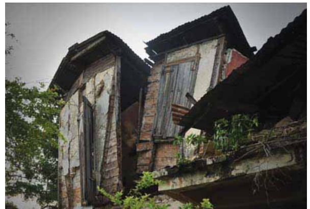
FIGURE 63 Heavily rotted and termite-eaten house on Avenue Lamartiniere, which partially collapsed during the earthquake.
