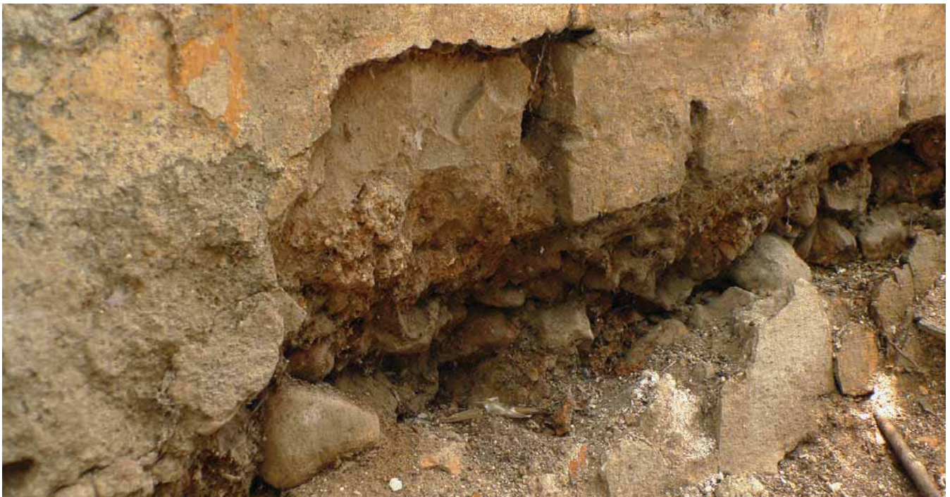
FIGURE 92 Basal erosion of the wall surface and foundation.
