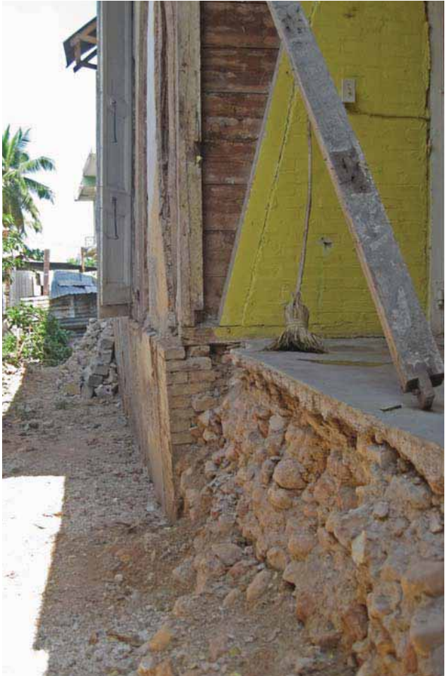
FIGURE 71 A portion of the foundation wall has collapsed at the house at 2 Avenue N, revealing that the crawl space below the first floor had been filled with rubble and the wood floor had been replaced with a slab on grade. Lateral loads on the wall from the fill caused it to collapse. The foundation wall remaining has rotated outward.
