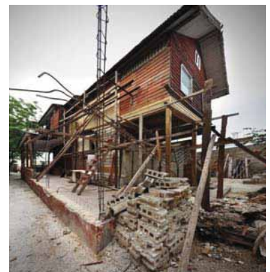
FIGURE 134 The modern reinforced-concrete frame with concrete-block back additions to the house at 24 Avenue Lamartiniere collapsed in the earthquake and have been removed. The owner, architect Gilbert Mangones, is now doing all of the repairs with timber framing and cladding, which will be much more compatible with the flexible timber frame of the original house, and less likely to collapse in a future earthquake.
