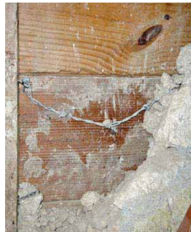
FIGURE 125 Barbed wire is frequently seen in the wall cavities as a restraint for the rubble fill. This is a good practice and should be continued.
