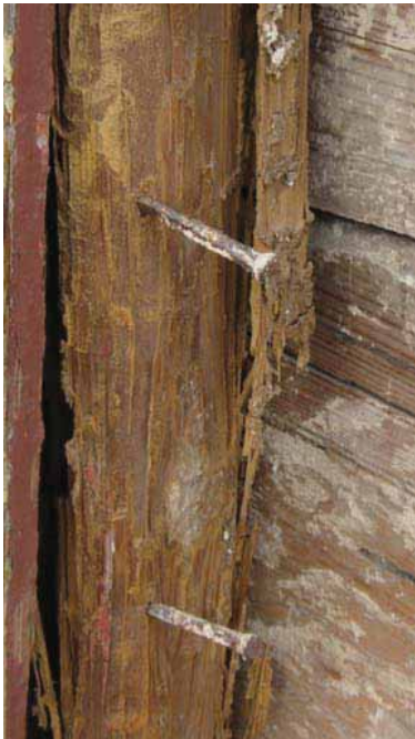
FIGURE 84 Despite extensive termite damage, the remainder of this post is hard and dense, still holding the nail firmly.
