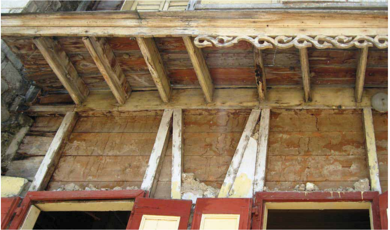
FIGURE 66 Poor construction and detailing have made many balconies vulnerable to decay and structurally unsafe. For those balconies supported on the cantilever extension of the floor joists, decay can extend into the house, putting both the balcony and interior floor at risk.
