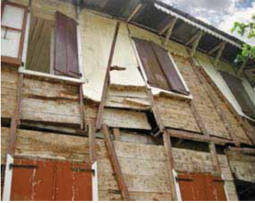
FIGURE 123 Typical vulnerability: the wall pulls away on the side parallel to the floor framing due to lack of connectivity between the floor and the wall. This is easily improved in most houses.
