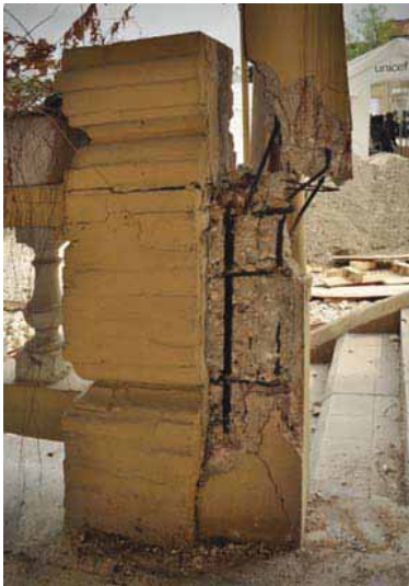
FIGURE 114 The Bazin House on Rue du Travail Deuxième. An upstairs bathroom of reinforced concrete and block construction clad with wood visible in the middle of the left photo almost caused the collapse of the entire house because it was standing on thin legs of heavily deteriorated concrete with rusted rebar. It was heavy, causing the whole house to sway, almost collapsing the bathroom wing, which may then have carried part of the house down with it.
