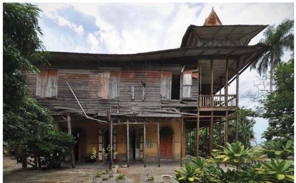
FIGURE 65: The Patrice Pamphile House (shown also in Figures 2 and 32) showing the heavily deteriorated wooden part of the structure, which at one time probably had been an open porch.
