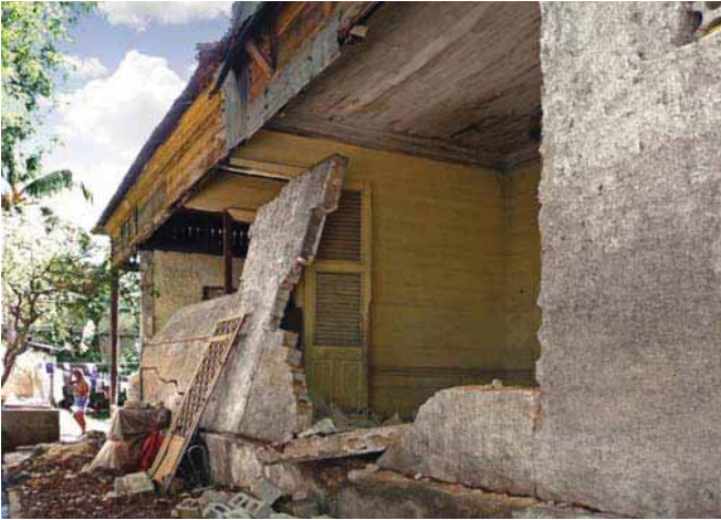
FIGURE 72 A replacement side wall of concrete block at 19 Lamariniere suffered partial collapse.
