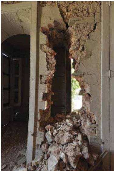
FIGURE 130 below left A rubble panel on the second floor of the Villa Castel Fleuri that collapsed showing the displacement of the bottom of the brick pier into the doorway which resulted from the expansion forces from the panel. below right Le Manoir on Avenue John Brown showing a heavy level of disruption of the masonry walls caused by the rapid degradation of the rubble stone panels during the earthquake.
