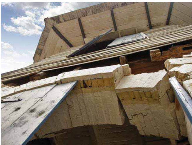
FIGURE 105 Severely damaged arch, and displaced wood framing above. Absence of tie rods, combined with decay of the timber sill plates made the building more vulnerable.
