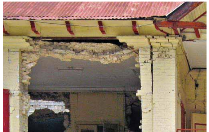
FIGURE 104 Total collapse was avoided in this heavily damaged masonry building due to embedded iron rods at the top of the walls, with exposed end plates.
