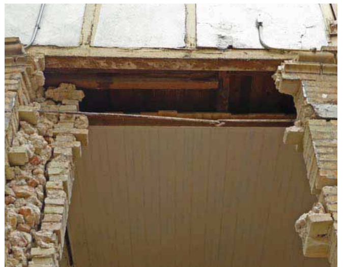
FIGURE 106 Linked iron tension rods exposed after the limestone infill panel was discharged. The rod may have prevented complete wall collapse.
