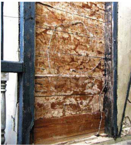
FIGURE 40 In this colombage construction the stone infill has collapsed due to the earthquake revealing the barbed wire reinforcement. This is an example of a non-construction material being adapted for construction due to its apparent availability. The barbed wire was galvanized and is still in good condition.
