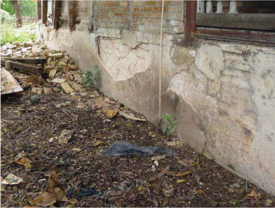
FIGURE 50 Spalling of the exterior finish plaster of the house at 84 Lamartiniere reveals two contiguous sections of foundation stem wall. One of irregular limestone left , and one of brick right .
