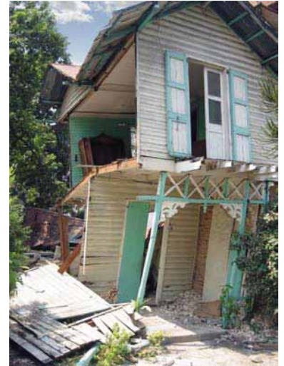
FIGURE 85 Despite severe damage, this timber frame building did not fully collapse. Note that the wall that fell away is the one on the side parallel to the joists, thus not having substantial tie to the floor.
