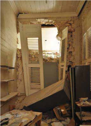
FIGURE 69 Hole in the masonry wall of Castel Fleuri caused by a concrete vault constructed in the exterior side and adjacent to this wall.
