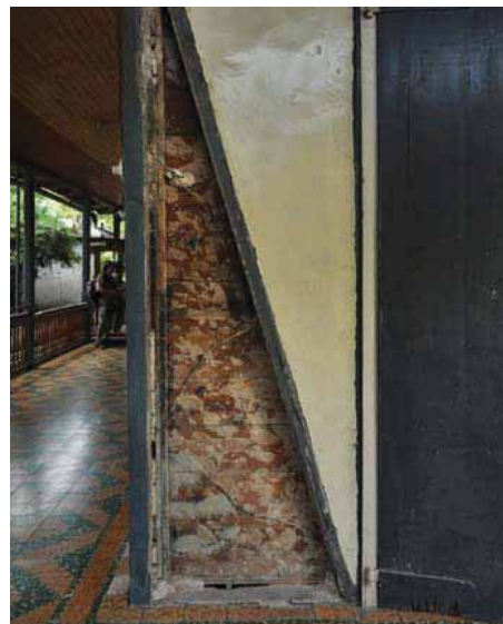
FIGURE 41 House at 15 Rue M showing plastered rubble stone infill. On the left, one panel fell out in the earthquake, revealing that it was reinforced with barbed wire inserted into the bay in a zigzag layout.
