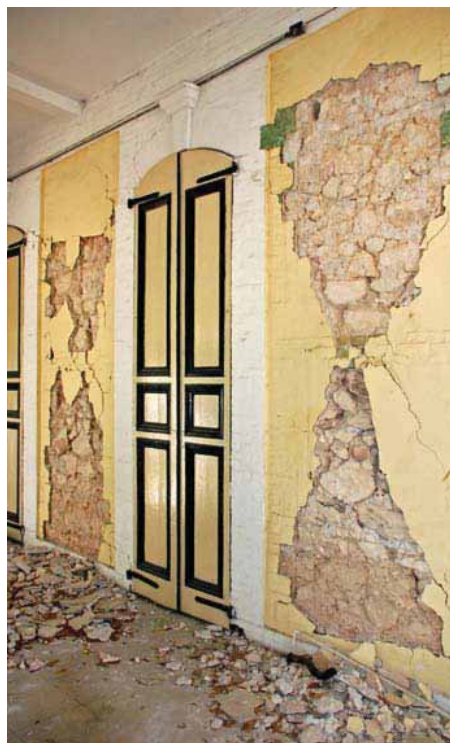
FIGURE 115 The characteristic X-cracks seen on masonry wall infills of concrete frames are also present at Le Manoir. These are due to the reinforced concrete second floor slab (above the damaged wall in this picture).
