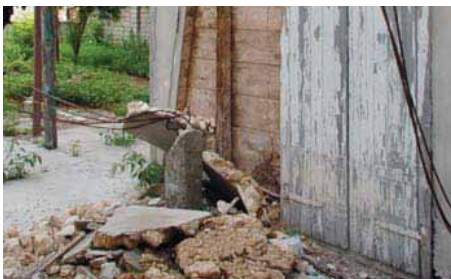
FIGURE 88 Stone infill that had been relaid with cement mortars would fall out of the wood frame in huge pieces during the earthquake causing damage also causing a safety hazard.
