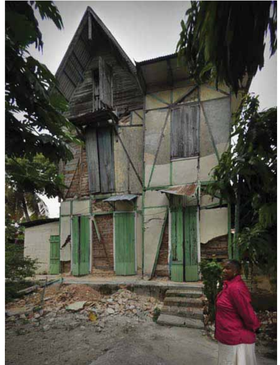
FIGURE 83 Marie Céleste Florence Jacob, seen here, continues to live in this century-old wood frame house at 14 Rue Marcelin. This house was extensively consumed by termites prior to the earthquake which damaged it further. Even in this badly compromised state, this structure remained standing after the earthquake only a few short blocks away from the National Palace and many other concrete frame structures which collapsed.
