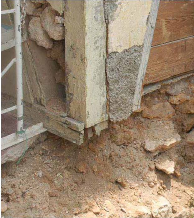
FIGURE 79 The wood sill that was previously termite damaged was crushed during the earthquake. This caused the entire structure to settle on its foundation. The result is that many of the doors to the exterior cannot be opened or closed.
