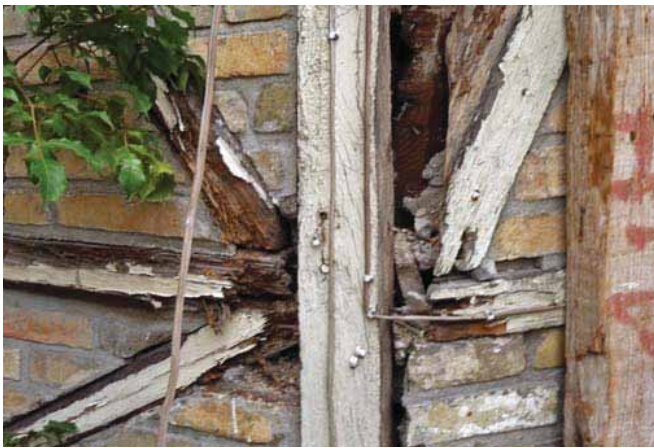
FIGURE 67 Rot of timber frame members at corner of colombage house at 32 Lamartiniere.
