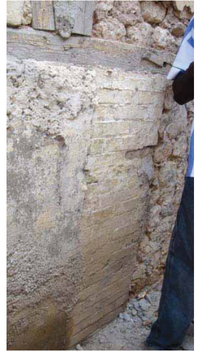
FIGURE 51 The original brick masonry foundation pier can be seen and is infilled on either side with stuccoed stonework. Rising damp from the ground has caused extensive deterioration to the exposed stone masonry. This results from the migration of soluble salts to the surface where they expand on drying, causing the surface of the masonry to spall.
