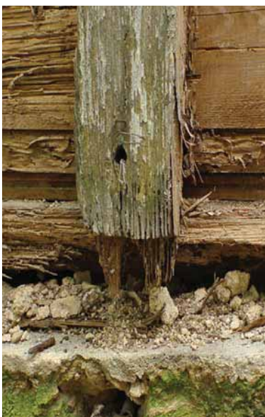
FIGURE 64 The post tenon is still present; the sill has rotted away.
