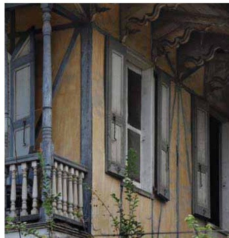
FIGURE 44 House at 15 Rue M showing undamaged second floor panels coated with a colored whitewash, giving an attractive patina to the surface of the stucco.
