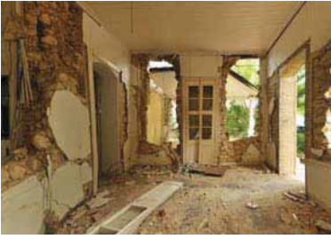
FIGURE 94 Ground floor interior of the Albert Dufort House on Rue du Travail Deuxième showing complete disruption of the rubble panels in its construction. The interior wall on the left, which did not have brick piers walls because of the lack of window and door openings, collapsed completely.
