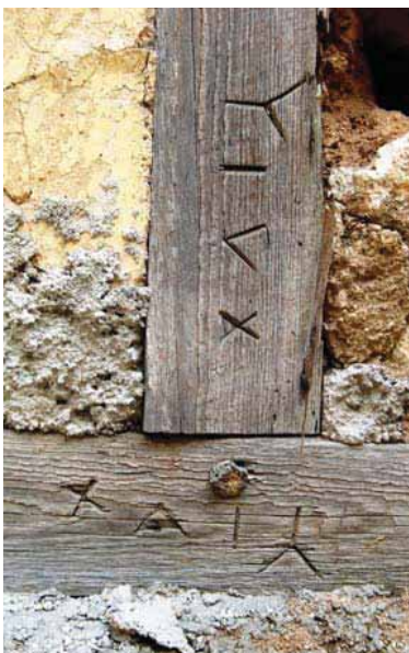
FIGURE 37 A detail of colombage construction. The wood frame is pegged with a trenail and the panel voids are filled with stone and lime mortar. The fill on the left still has the clay stucco in place. Note the carpenter's marks carved into the wood members.
