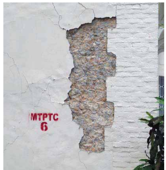
FIGURE 4 The red painted designation “MTPTC” indicates that inspection deemed the tower unsafe for occupancy by the Ministère du Travail Public et Télé Communications.
