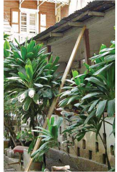
FIGURE 119 Temporary measures are important: this lateral brace is a good idea, but it is too slender and there is only one.
