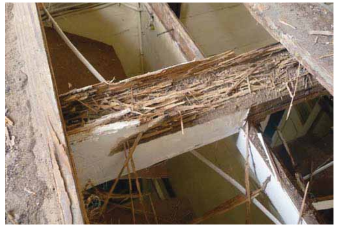
FIGURE 68 Termite damage in second story floor joists.
