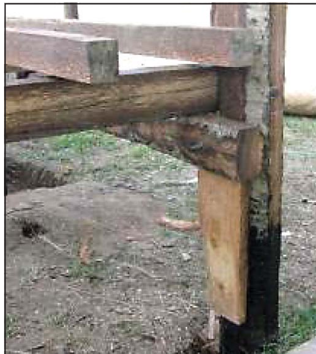
Cross joist and long joist mounted on post with nuts & bolts and cleat ▲
