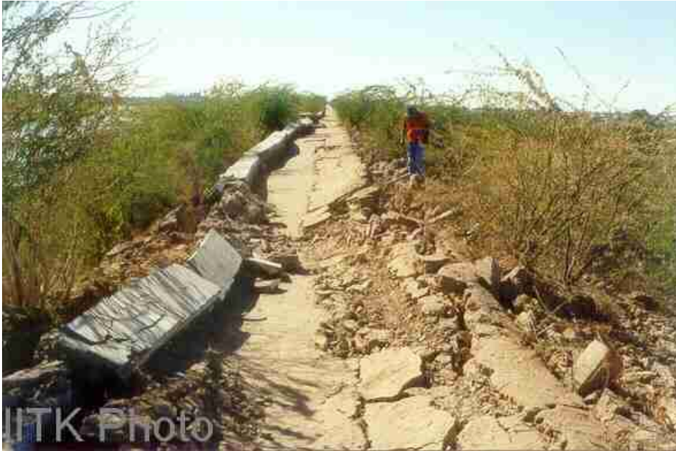
Cracks along the crest and vertical settlement of the Suvi dam.
