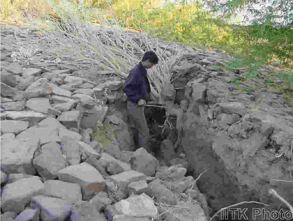
Massive cracks in the upstream embankment near the toe of the Fatehgadh dam.
