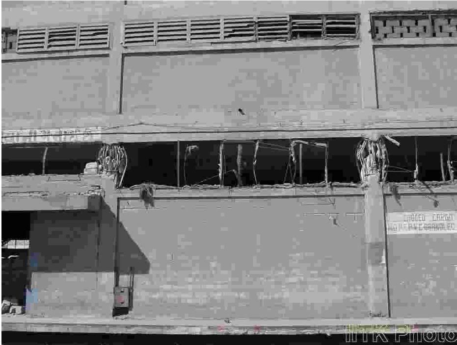
Severe damage (cyclic shear cracks) to the exterior short columns at the ventilators of the warehouse at Kandla port; opening of ties and buckling of longitudinal steel.
