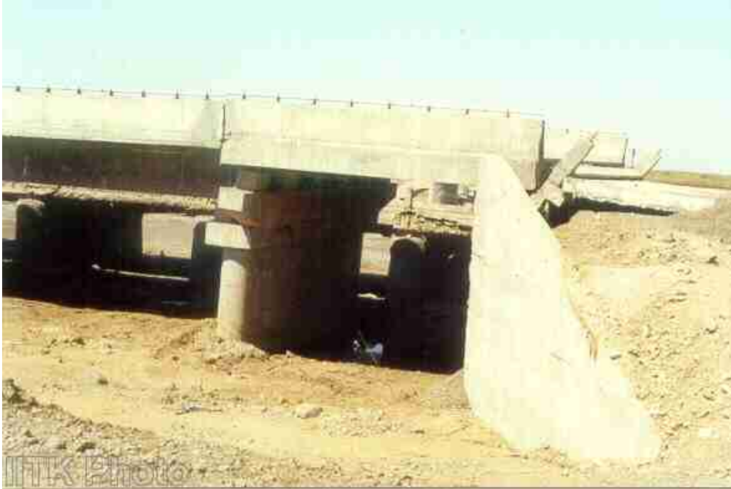
Lateral movement of soil at the abutment of the four-span RC bridge near Vondh.
