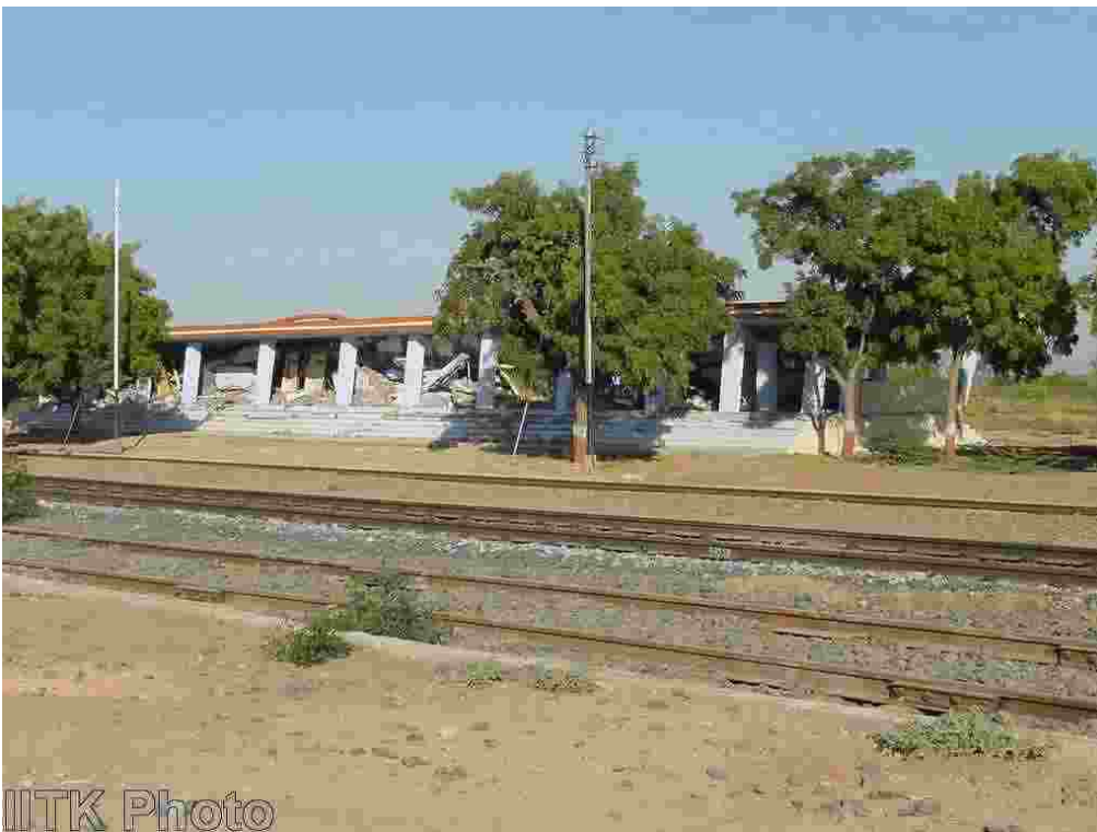
Collapse of the brick masonry railroad station building at Vondh.
