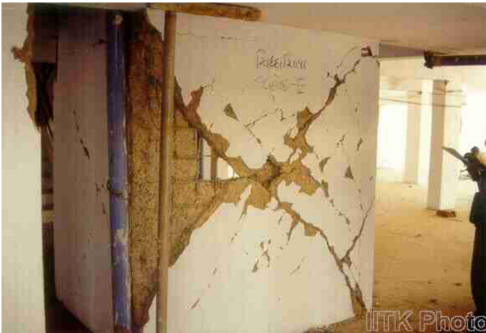
Severe shear cracking sustained by the RC elevator core wall in a four-storey RC frame building in Ahmedabad.
