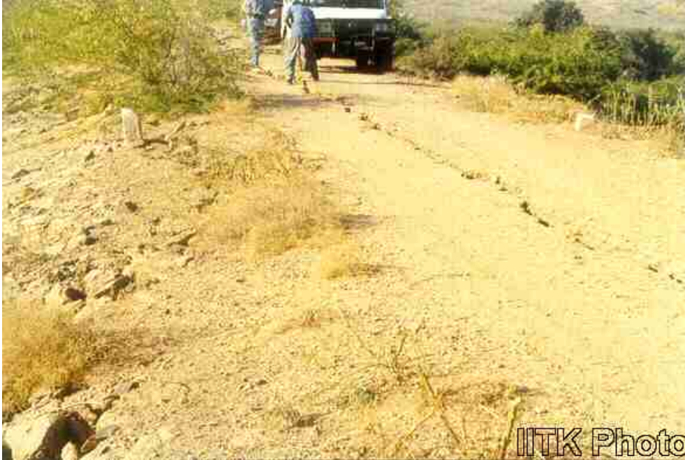
Longitudinal cracks along the crest and the downstream slope of the Kaswati Dam.
