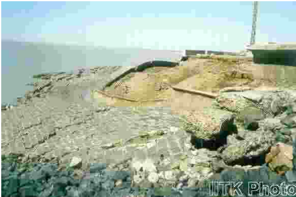
Failure of sea wall at Navlakhi port; over 50 meters stretch of the wall was washed away into the sea.
