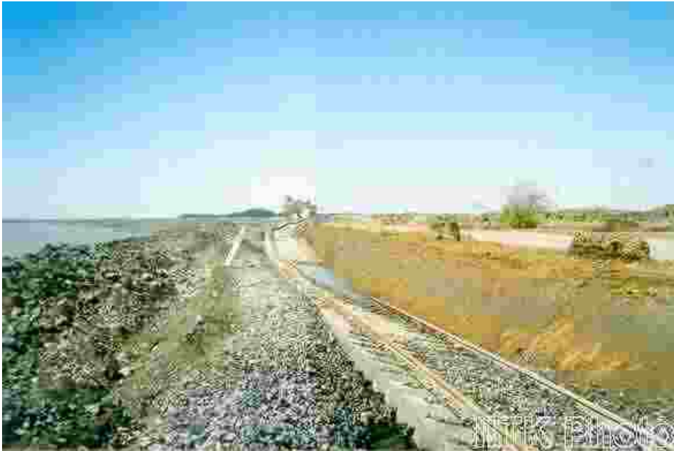
Massive slope failure of the rail-road embankment near Navlakhi port resulting in fracture of rails, and damage to prestressed concrete sleepers and panroll clips.
