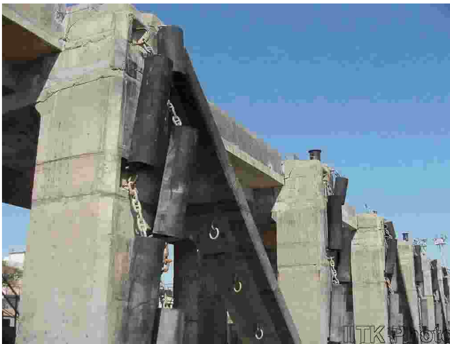
Flexural and shear cracks at the beam-column joint at the knee-bent frame supporting craft jetty at Kandla port.
