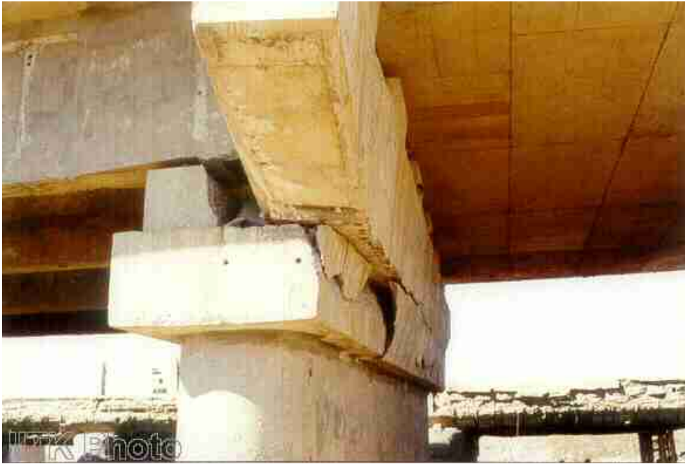
This pier at the RC bridge near Vondh was found to have a tilt. Considerable liquefaction was observed at the site.
