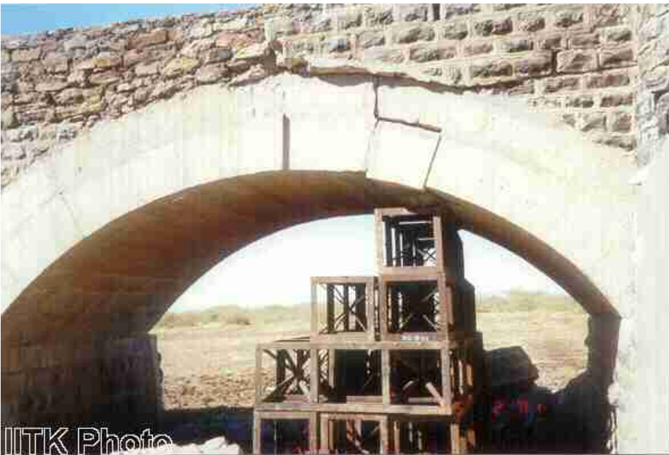
Unsymmetrical failure of stone masonry arch railway bridge.
