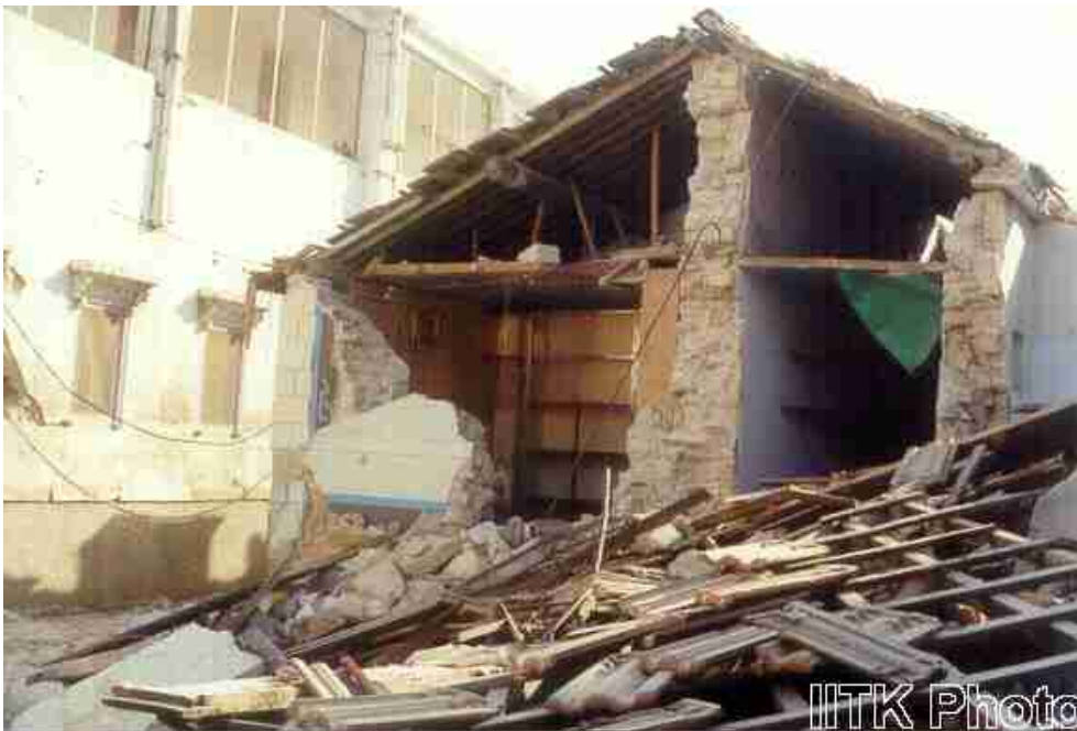
Out-of-plane collapse of masonry wall.
