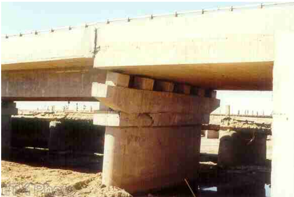
Damage to the unequal-height bed blocks at the RC bridge near Vondh. The pier supports two spans with different girder/slab depths.
