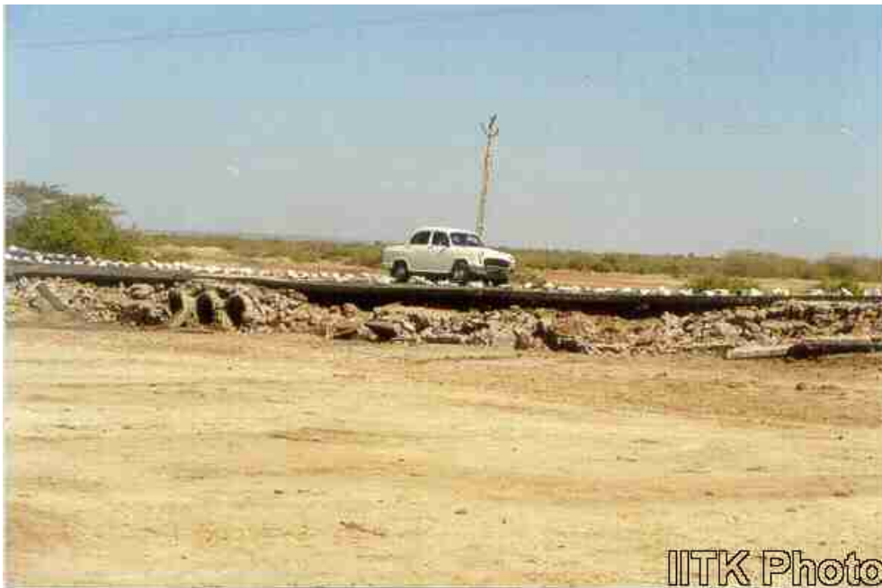
Damage to pipe culvert. The site had considerable liquefaction.
