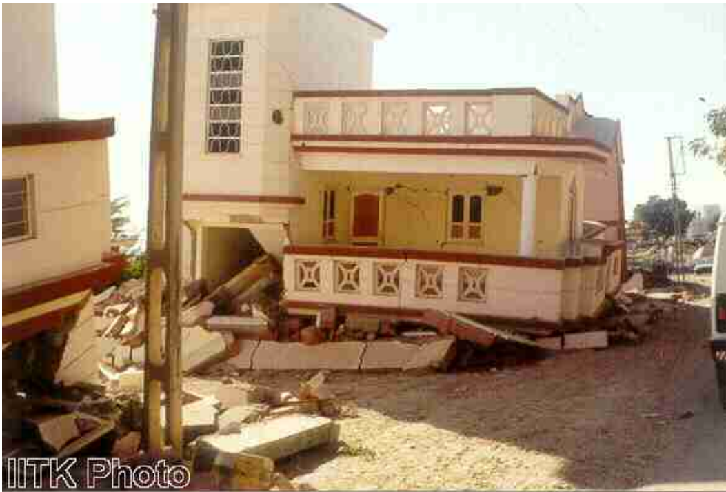
Collapse of ground storey of a two-storey RC frame building in Manfara village.
