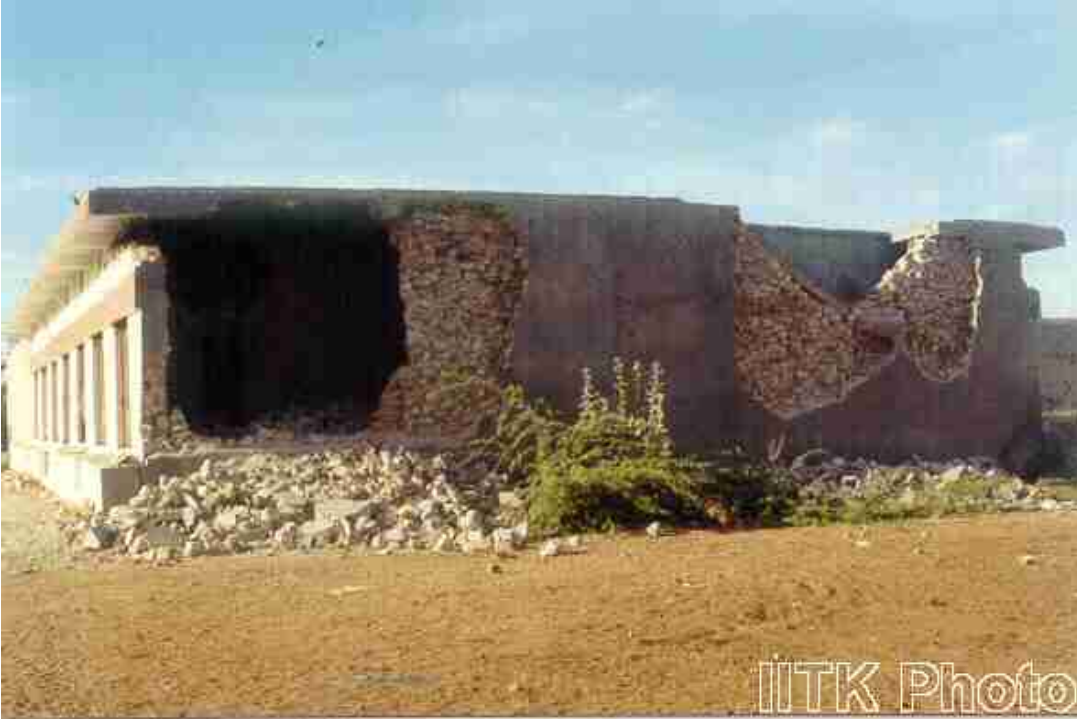
Uneven out-of-plane collapse of the wythes of the stone masonry walls in single-storey building with RC slab roof near Ahmedabad.
