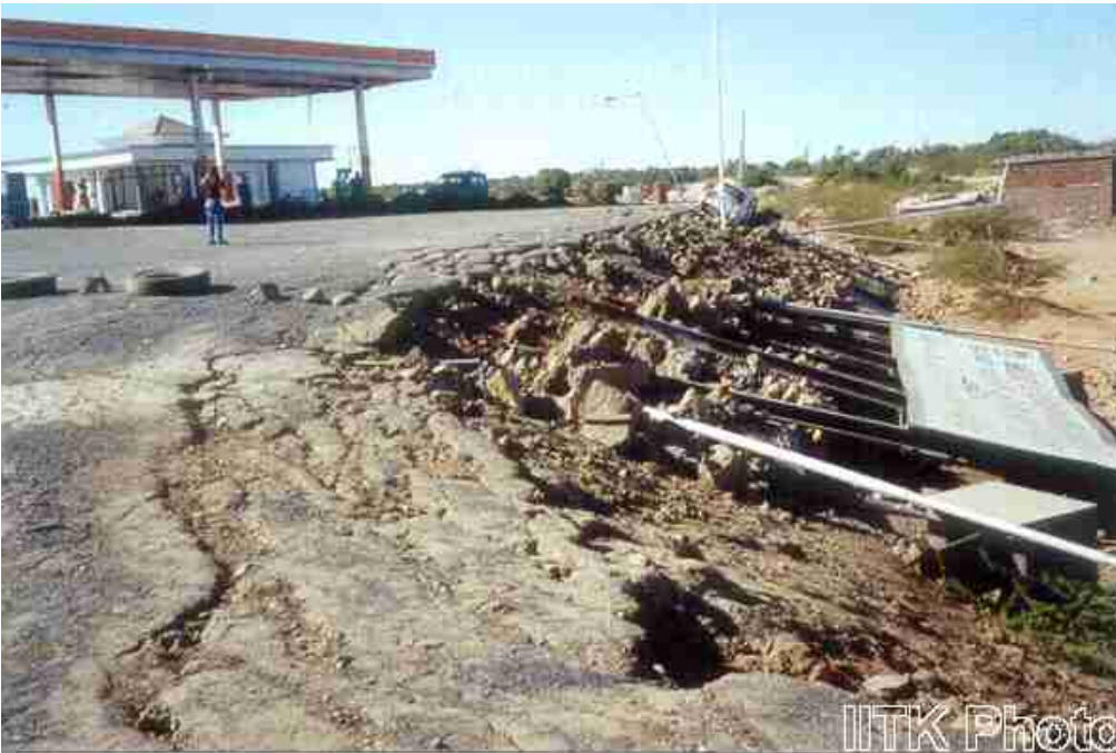
Damage to kerb of highway pavement due to lateral spreading of soil.
