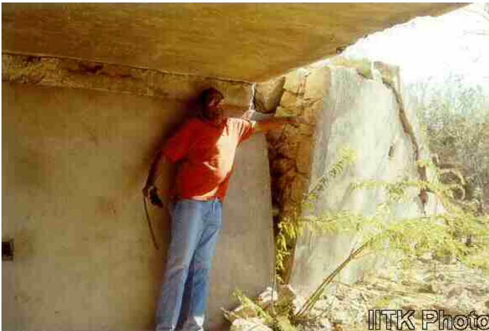
Lateral movement of the wing wall at the abutment of RC slab bridge.
