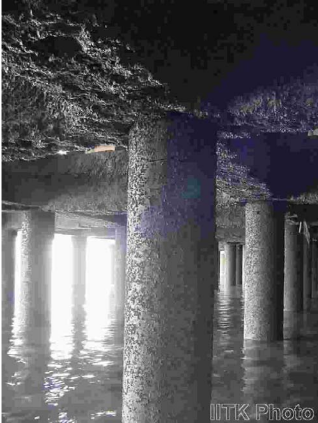
Flexural cracking of the piles at the jetty at Kandla port.
