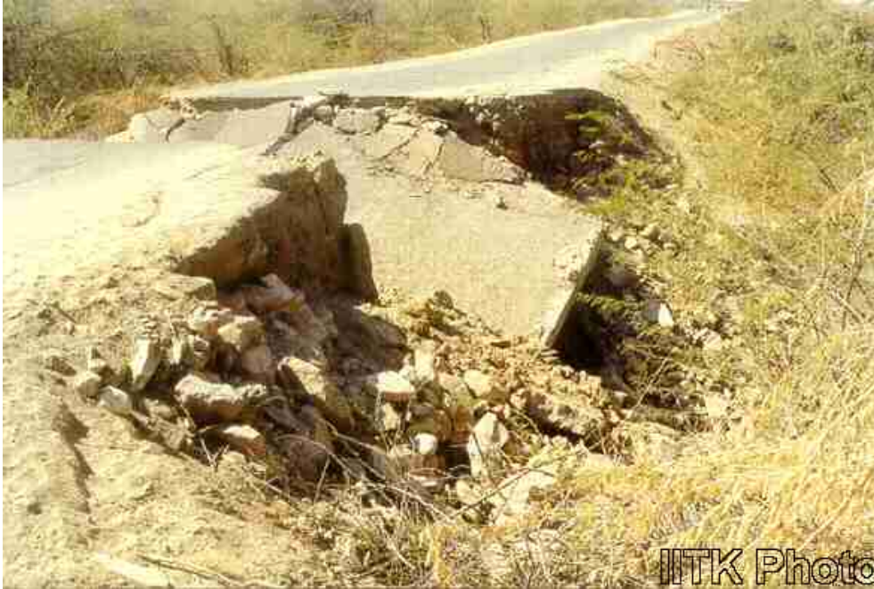
A number of RC slab culverts on stone masonry abutments sustained damage.
