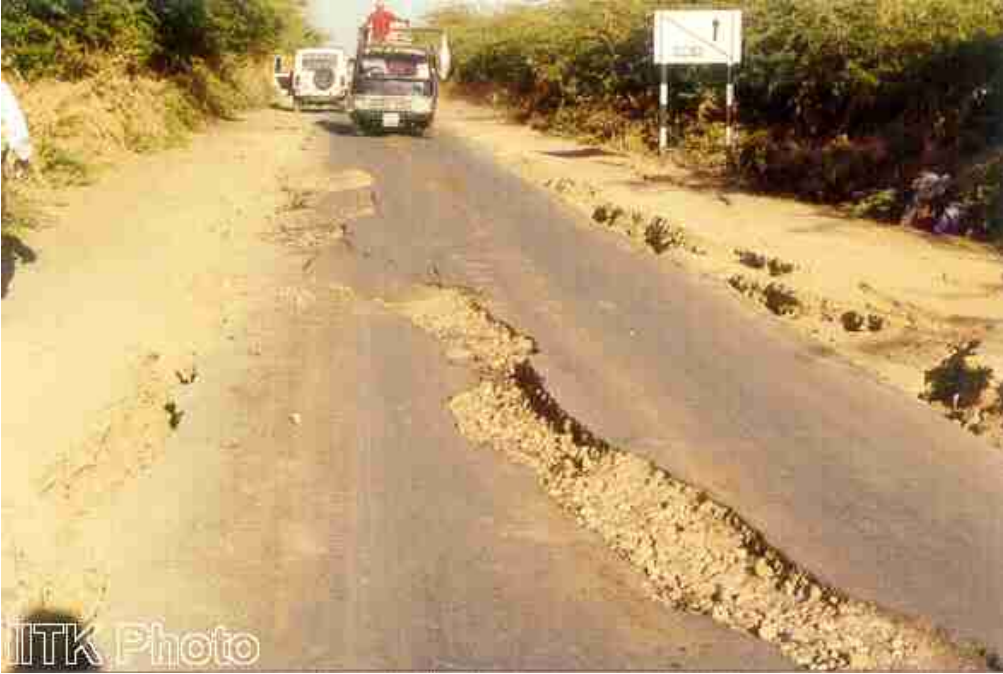
Damage to highway pavement near Rapar due to lateral spreading of soil.
