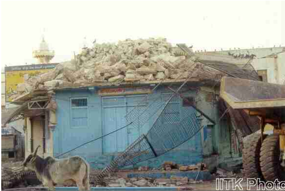
Collapse of upper storey of a commercial building in old Bhuj.
