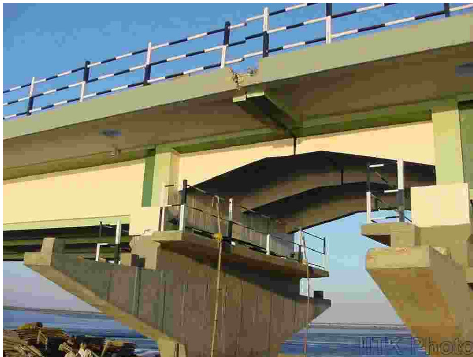
The longitudinal movement of the new Surajbadi bridge superstructures led to pounding at the deck slab level.
