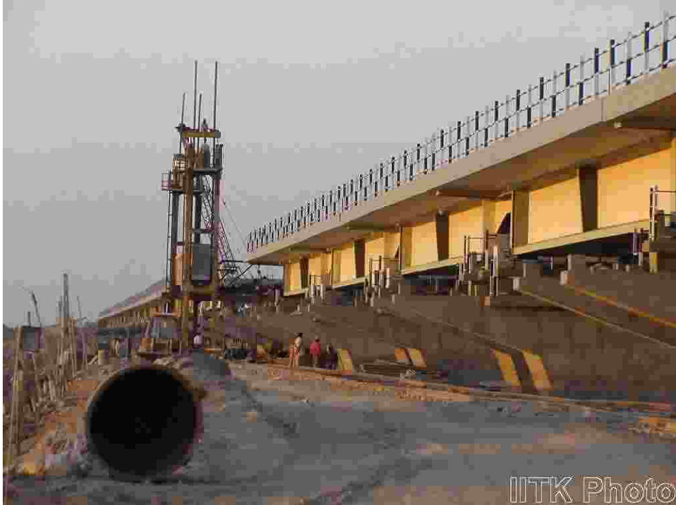
Prestressed concrete girder bridge nearing completion at Surajbadi. Completed spans sustained substantial damage like pounding of the deck slab, horizontal movement of girder, and damage at the bottom of girders.
