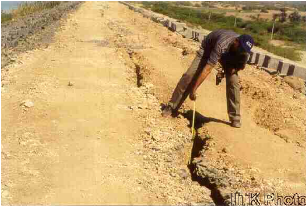
Cracks along the crest of the Tappar Dam
