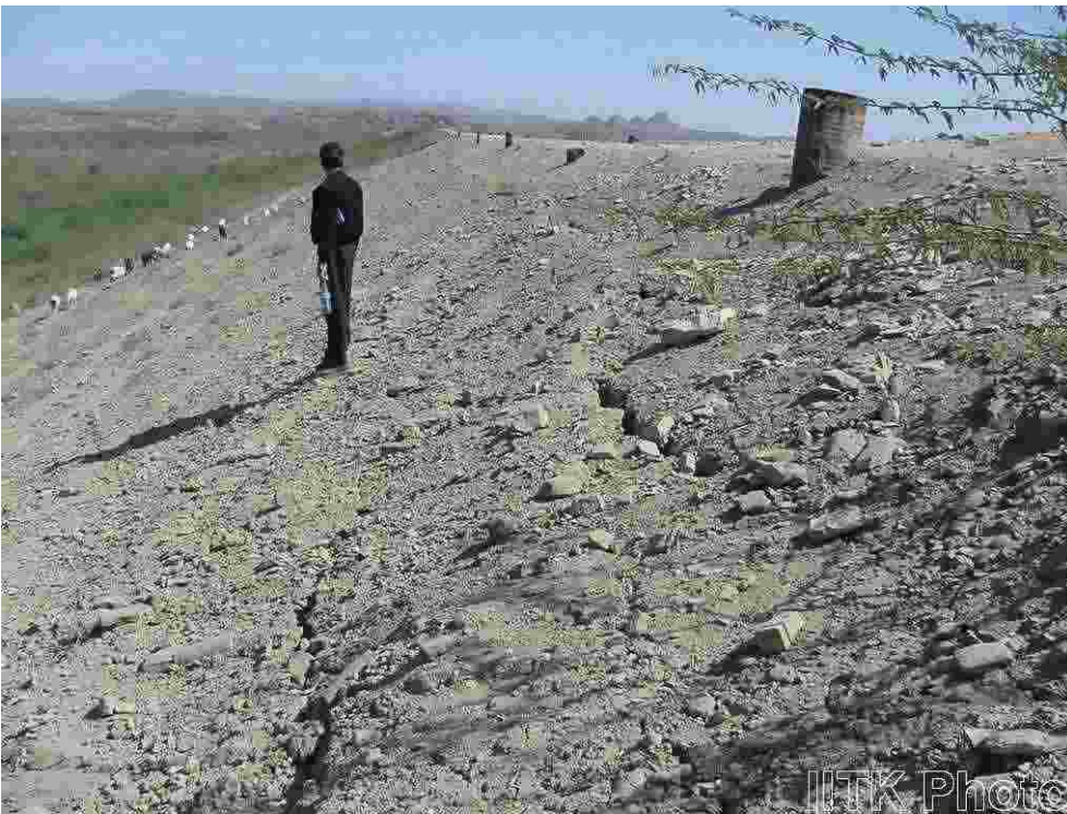
Lateral spreading of the downstream section of an earthen dam at Rudramata.
