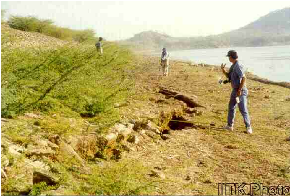
Lateral spreading at the toe of the Kaswati Dam.
