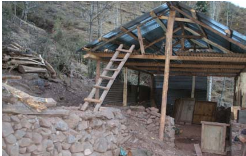
Reconstructing houses in an earthquake-resistant way is one method for sustainable recovery.
