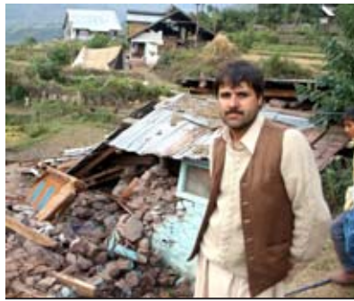
The poorly constructed house of an earthquake victim in Kashmir 2005 reflects poverty.
