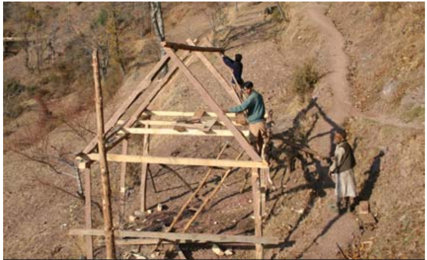
Affected people constructing their new houses, participating in the cash for shelter programme.
