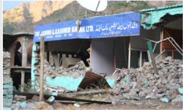
Public as well as private infrastructure suffered severe damage.
