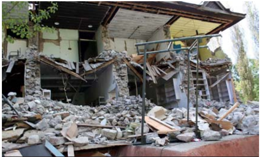
Damage and destruction due to the earthquake in Uri block of Baramulla district of Kashmir.
