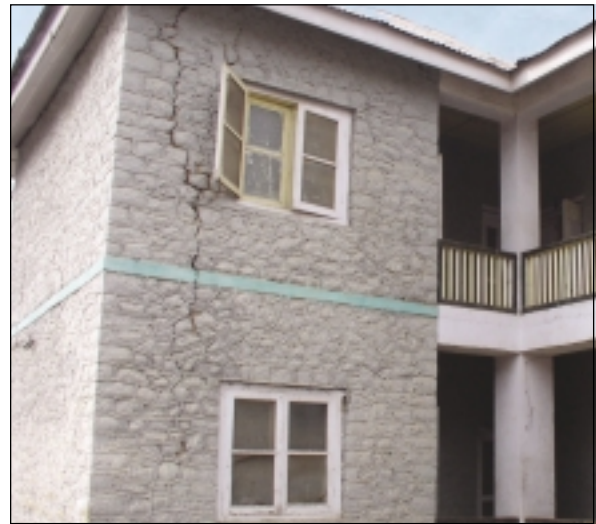
G3 damage crack in random rubble wall
