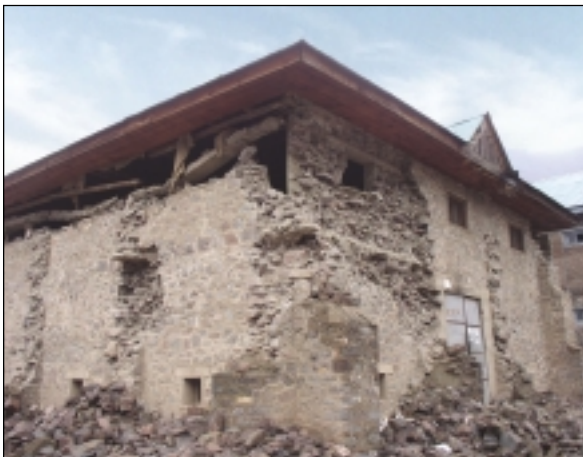
Damaged portions of walls need to be repaired and rebuilt
