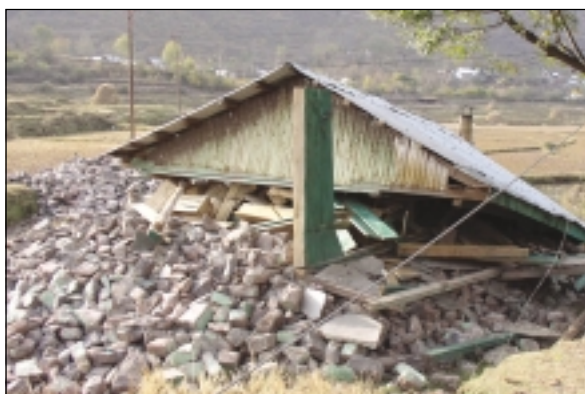
G5 damage, total collapse
