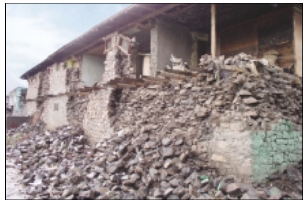
G5 damage in random rubble wall
