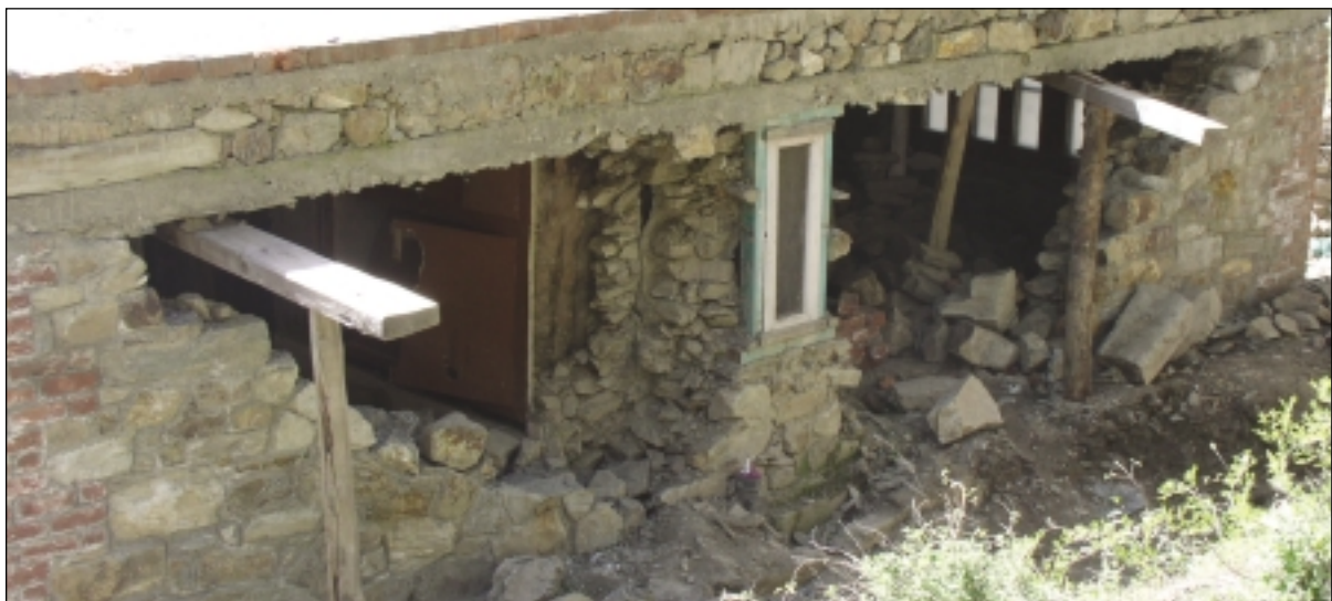
Undamaged RCC roof with badly damaged support walls
