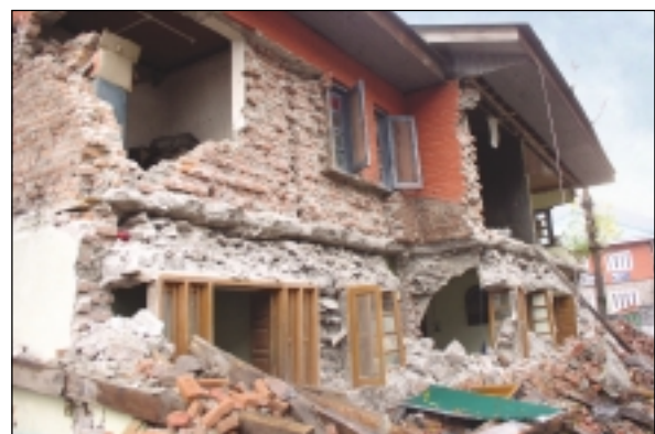
G5 damage walls heavily damaged, roof intact
