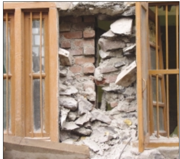
G4 damage in combination of stone and brick wall
