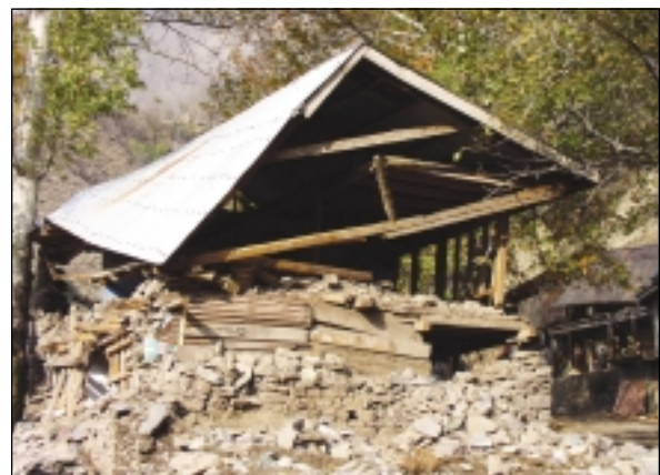
Tilted roof because of wall collapse
