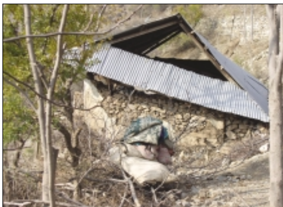
Tilted roof because of partial wall collapse
