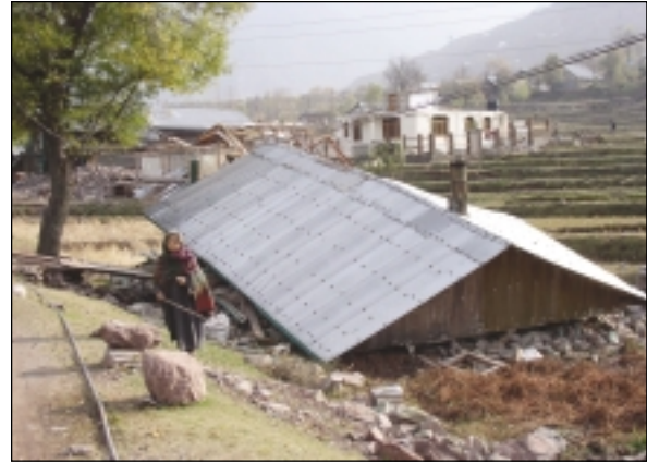
Roof slid down because of total wall collapse
