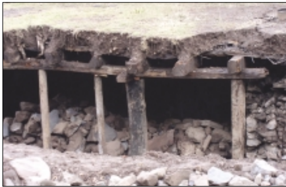
G5 damage in traditional mud roof building
