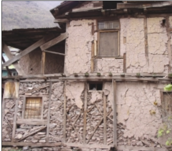
Minor damage to Dhajji wall - Cracks in in-fill
