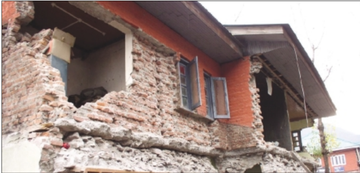
Wall damaged due to in-adequate bonding between brick masonry walls and roof deck
