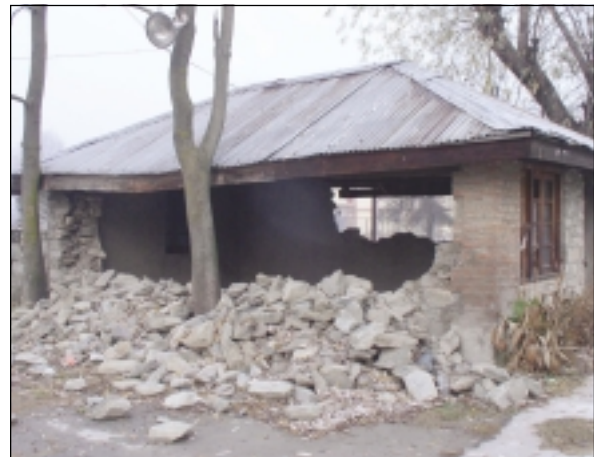
Roof needs to be jacked up, collapsed portion of walls need to be rebuilt
