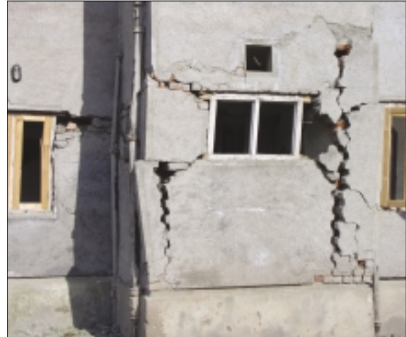
Damage due to inadequate in-plane tensile strength
