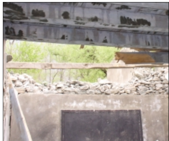
Breaking of timber floor under the impact of collapsed wall
