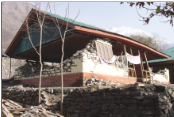
G5 Damage, severely damaged walls with damaged roof in place
