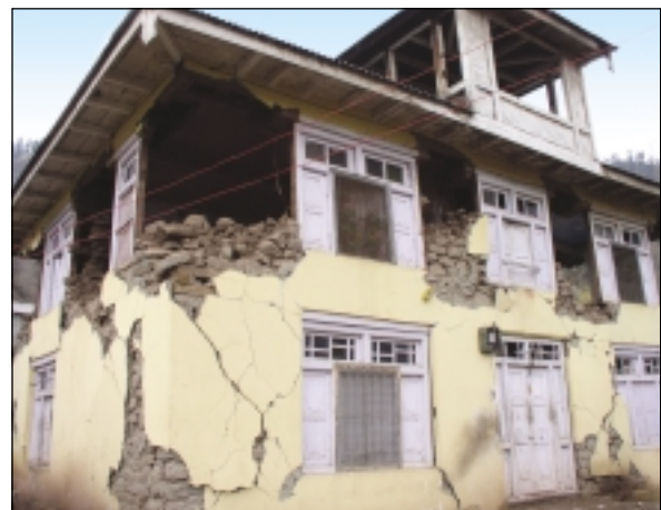
The roof, intermediate floor and ground floor walls including the foundation can be salvaged while rebuilding collapsed walls and repairing damaged ones
