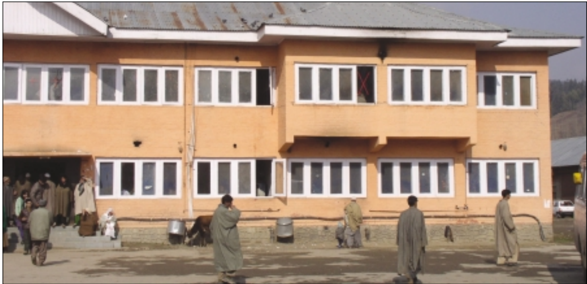
Existing building - large numbers of window openings in walls make it vulnerable
