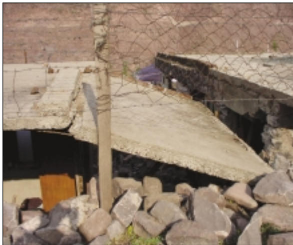
Slab failure due to collapse of support wall
