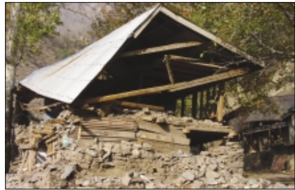
G5 damage in random rubble walls and CGI roof
