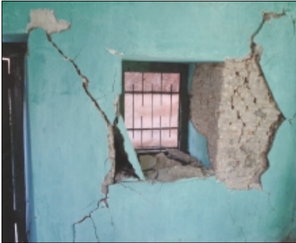
Diagonal cracking; pier width too small
