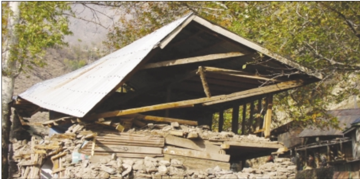
Roof damage due to inadequate in-plane strength
