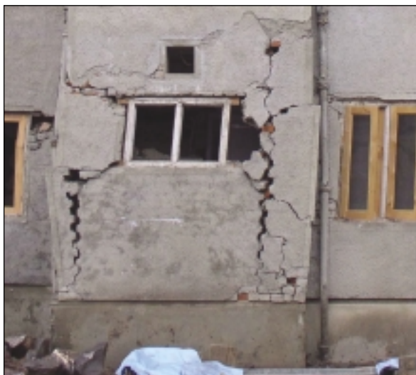
G4 damage cracks in brick wall
