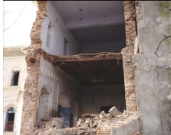
Poor storey-to-storey bonding
