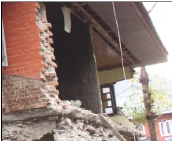
Poor wall-to-roof bonding
