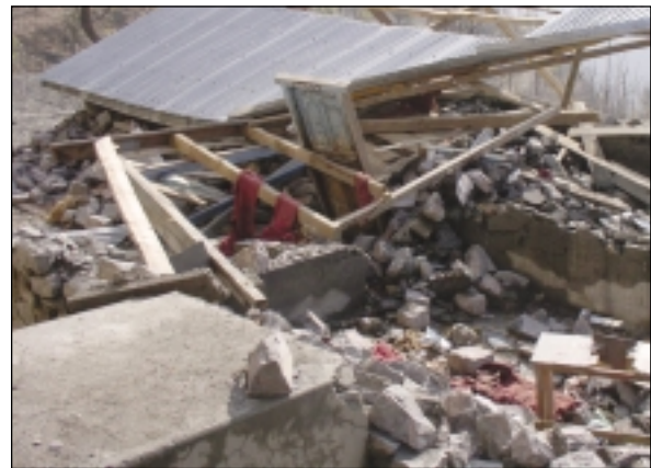
Roof destroyed due to wall collapse
