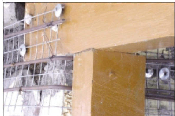
Belt continuity at corner behind wood post obstruction
