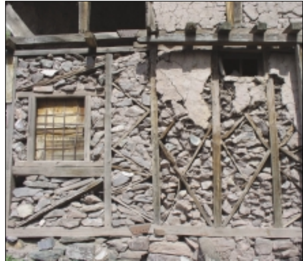
Chunks of plaster popping off exposing lack of horizontal bracing and loose in-fill masonry
