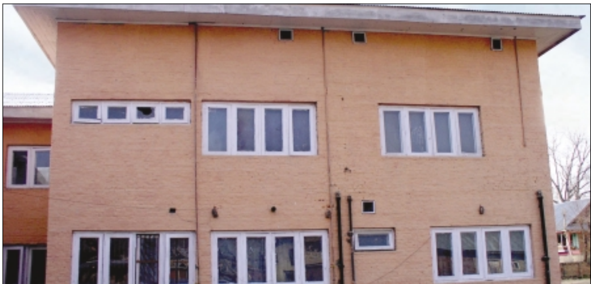
Existing building - exceptionally high walls make it vulnerable
