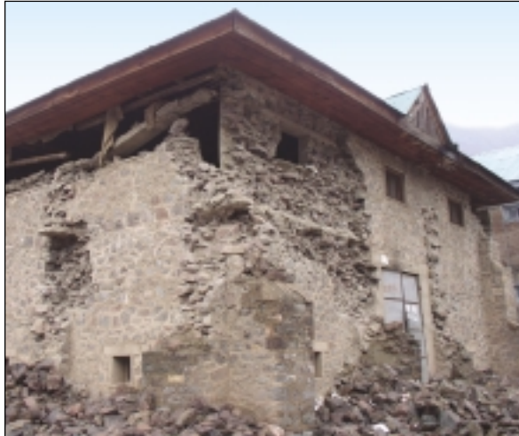
Damage in extra long wall
