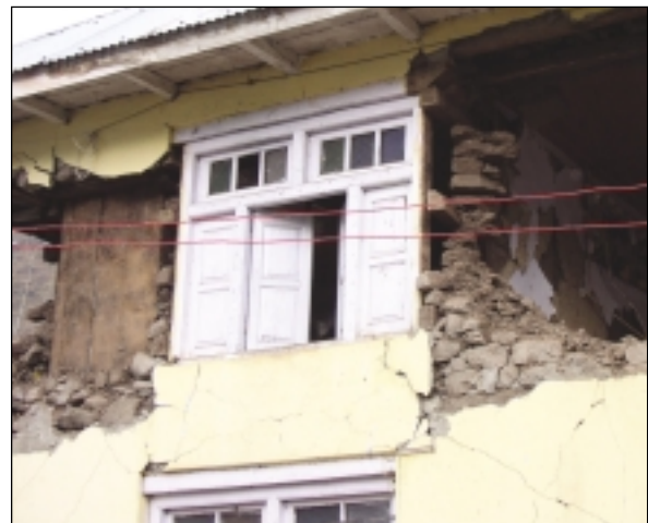
Poor wall-to-roof bonding
