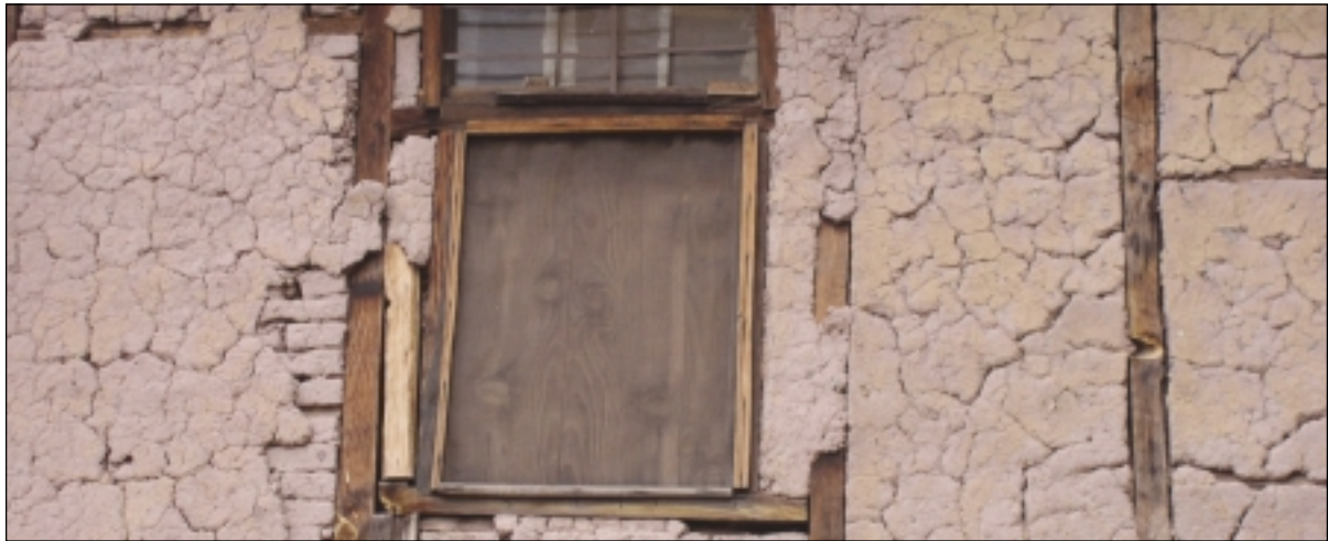
Popping off of plaster
