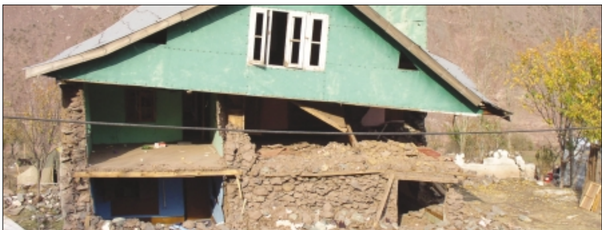
G5 damage in random rubble wall
