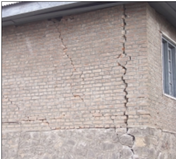
G3 damage crack in brick wall
