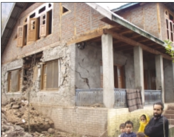
Damaged walls need to be restored
