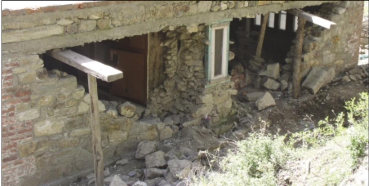
Undamaged RC slab on severely damaged wall
