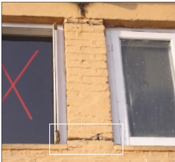
Damage: Pier failure
