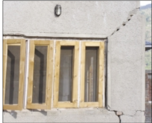
Severe diagonal cracking; windows too close to corner
