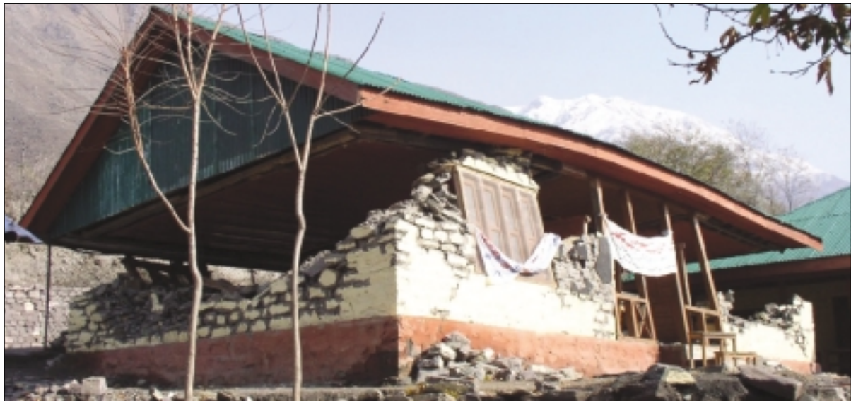
Damaged RR walls due to in-adequate bonding between roof and walls
