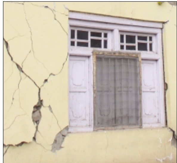
Diagonal cracking in RR wall
