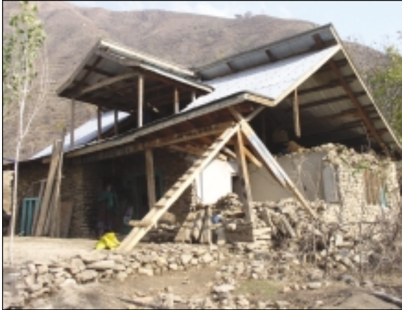
Collapsed walls need to be rebuilt
