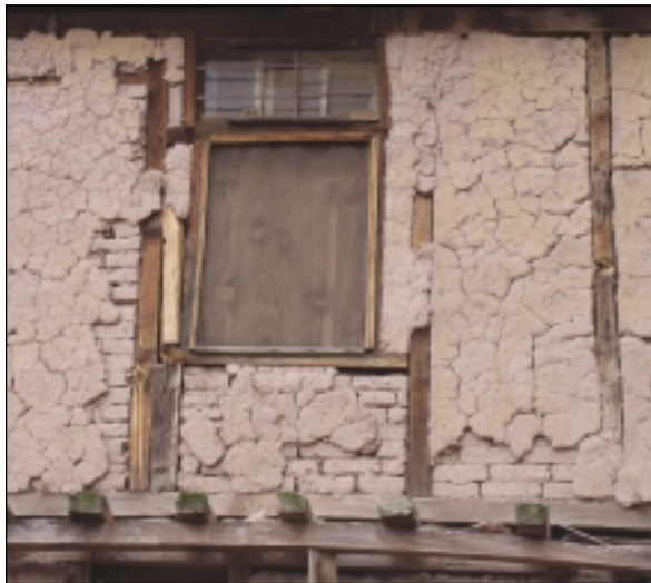
Minor damage in Dhajji wall
