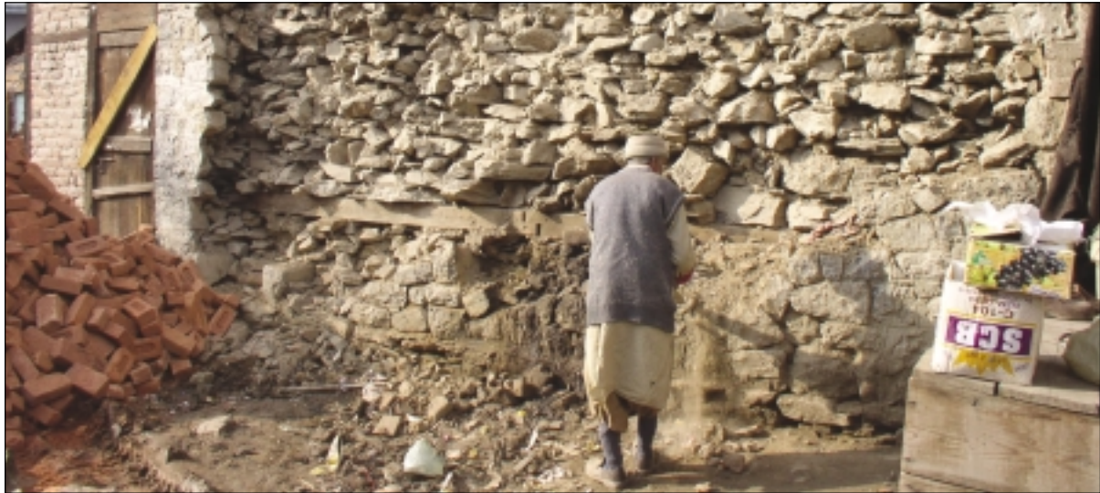
Delamination of wythes
