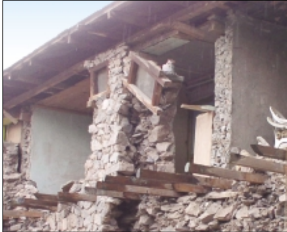
Inadequate bending strength in masonry
