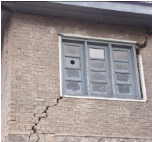
Diagonal cracking in brick wall
