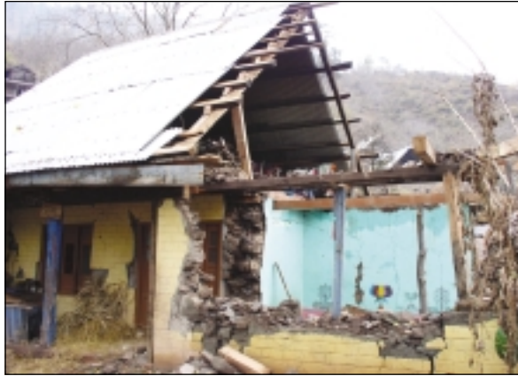
Collapse of roof because of wall collapse
