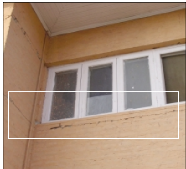
Typical damage at opening
