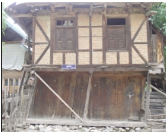
In-plane deformation - tilting of timber frame
