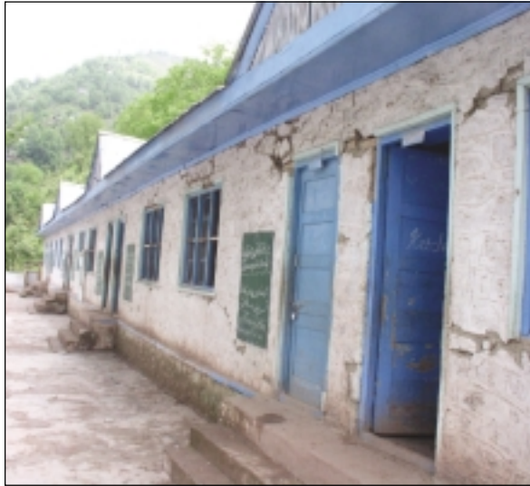
School with wall having G2 cracks
