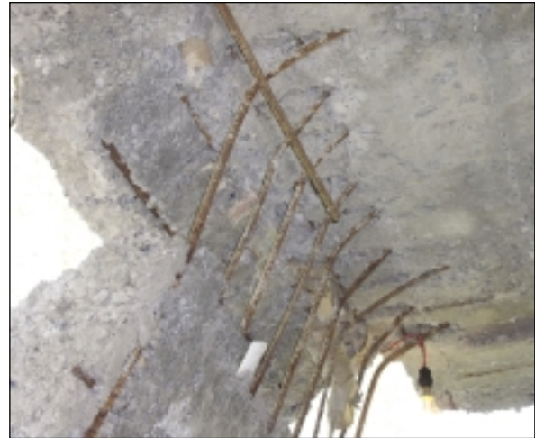
Wrong rebar arrangement at stair causing damage
