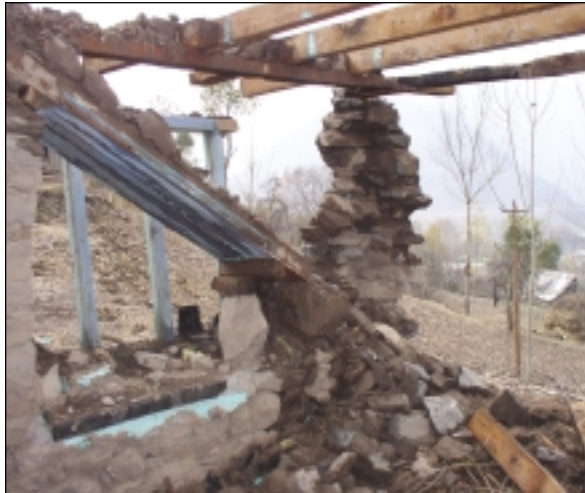
Snapping and collapse of timber floor joists
