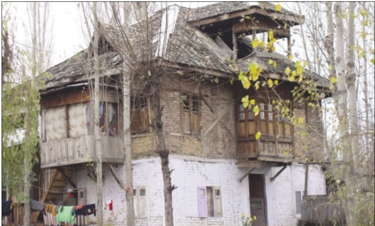
Wood shingle roofing on timber placed on brick masonry and dhajji walls
