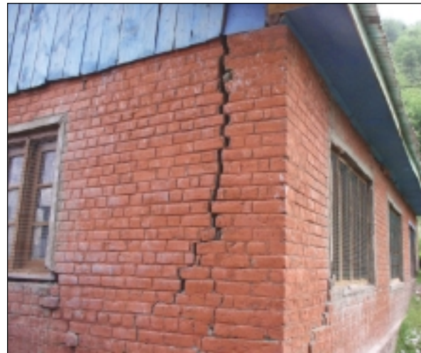
Damage due to poor wall-to-wall bonding
