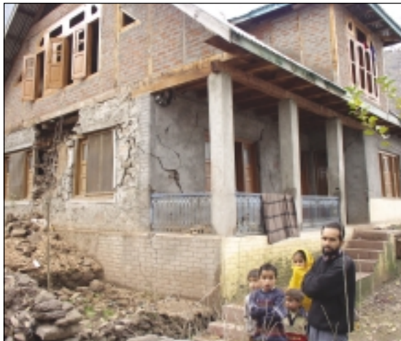
Damage in extra high wall
