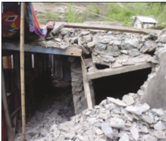
Collapsed support wall causing snapping of timber floor elements
