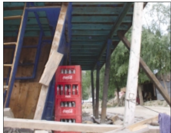
Swaying of timber frame with tilting of timber posts
