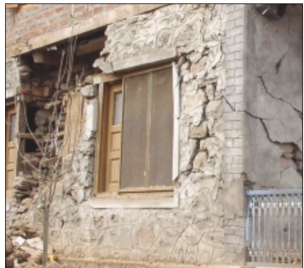
G4 damage in random rubble wall
