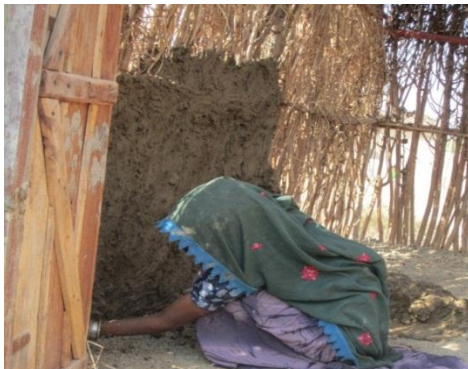
Champa, wife of Heero, Mir Khuda Bux village, plastering the walls of her shelter. Photo: Áine Fay, Concern. January 2013
