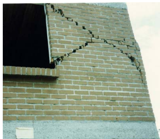
Figure 8. Shear failure due to wall stiffening.
