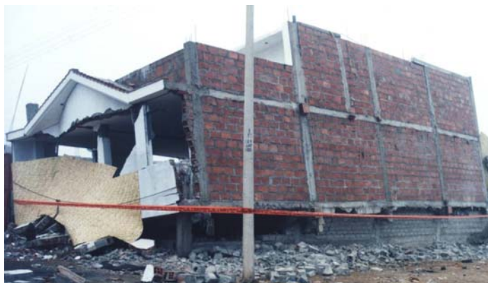
Figure 3. Collapsed house in the Atico earthquake.
