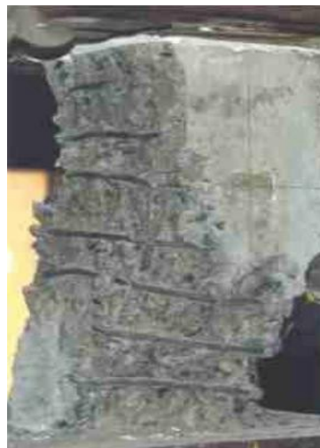
Figure 15. Concrete cover spalling and undamaged concrete core.
