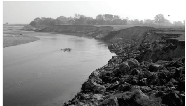
Figure 4-2: Typical Bank Erosion by Riverine Flooding
