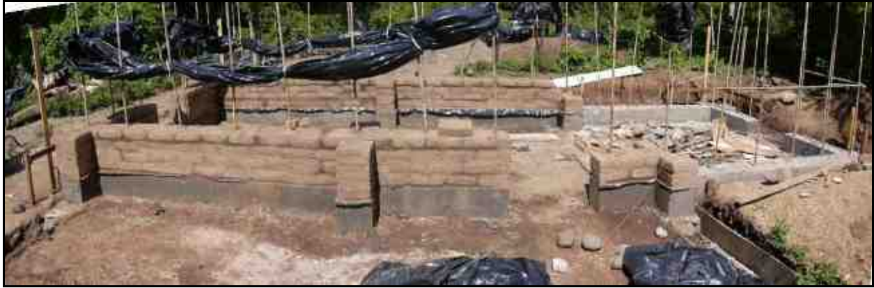
Figure 5. Adobe walls under construction, including plinth, pilasters, vertical reinforcement, plastic rain covers (Note: figure alignment offset due to photograph splicing).
