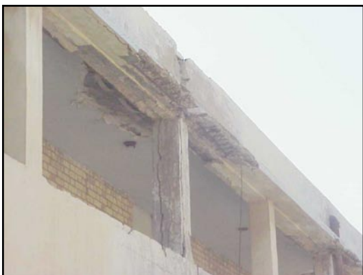
External Wall's Damages
