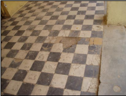
Damaged cement tiles in a classroom
