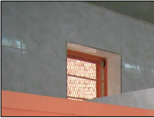
Toilet's door in bad condition
