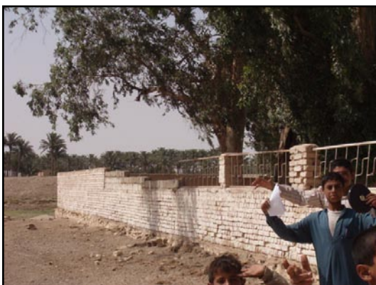
A school fence in bad condition
