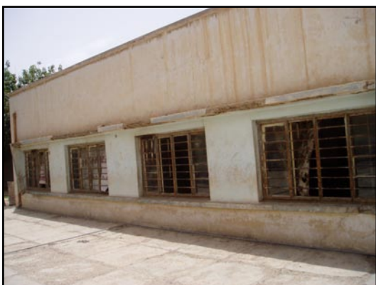
External walls of bad condition
