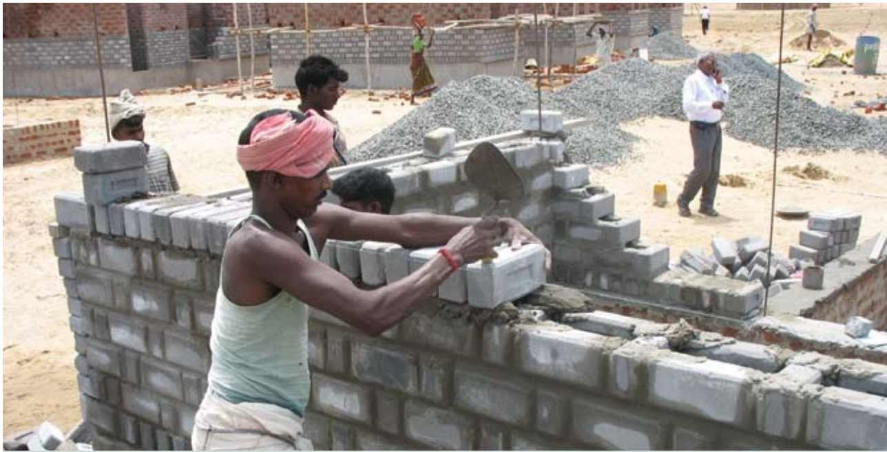
'Rat trap bond' masonry is a cost-effective method, reducing consumption of bricks and mortar.
