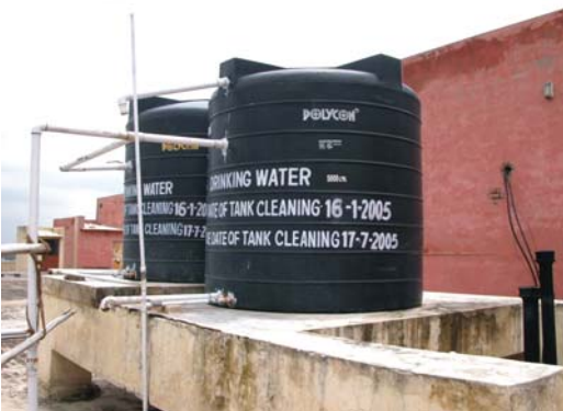
Syntex Water tank at roof without anchorage
