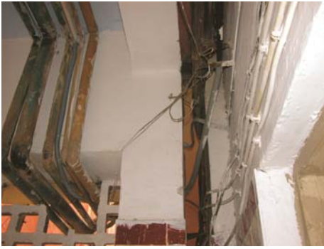
Pipes crossing an expansion joint on buildings: no flexible connection.
