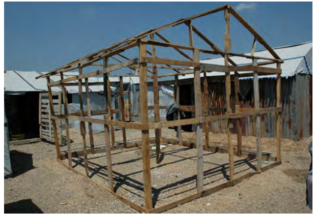
New shelter showing typical timber section sizes and spacing. Rudimentary wall plate and base plate for continuous fixing of plastic. Pitched roof.
