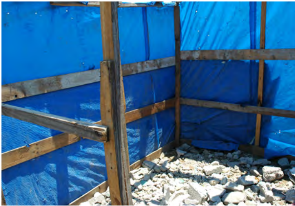
New shelter under construction, showing recycled roof battens and wooden pallet timber used for framing. Usually no bracing in the wall or roof frame.
