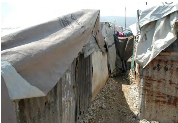
Good quality shelter grade plastic over self made shelter, used for roofing as waterproofing priority. Plastic damaged due to inadequate fixing.
