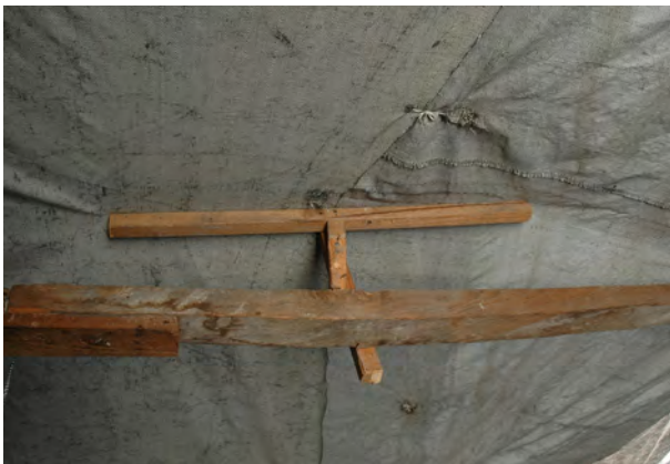
Small pieces of timber used to raise the centre of the roof to provide a fall for drainage on an shelter with a flat roof.
