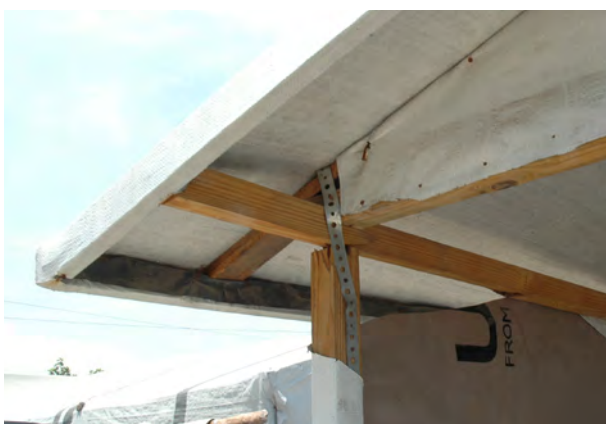
Hurricane strap used to tie roof trusses to posts. Ties, timber and carpentry support provided in reinforcement programme.
