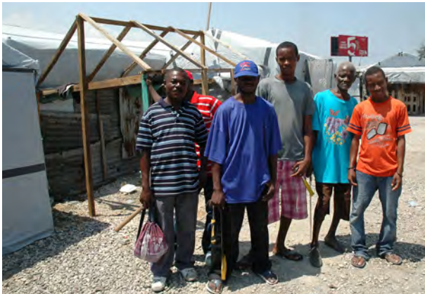
IFRC technical support team, carpenters from the camp, employed to improve all makeshift shelters, minimal material support, priority was weatherproofing.
