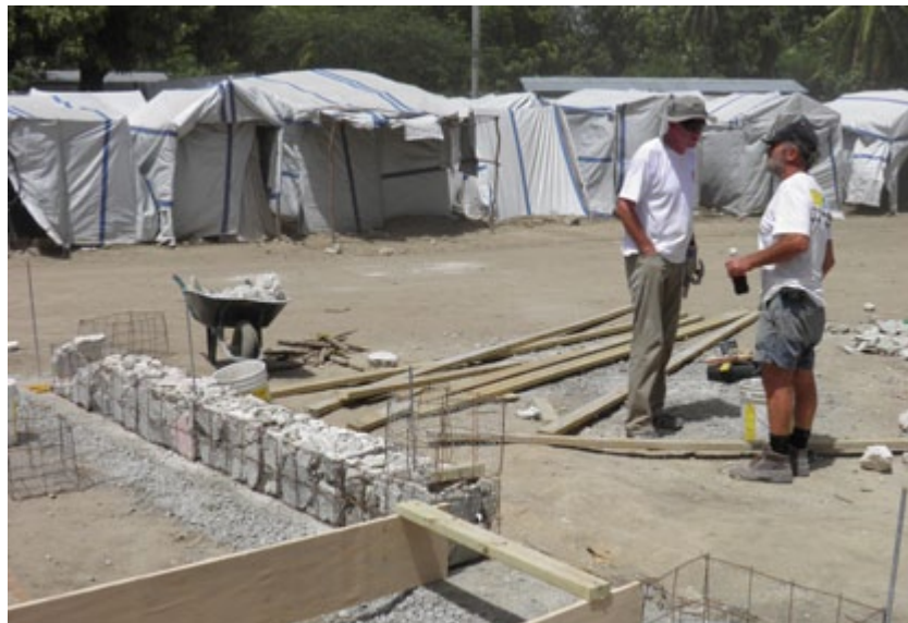
The debris advisor works on the construction of a Gabion-based house with a shelter agency in Haiti.
