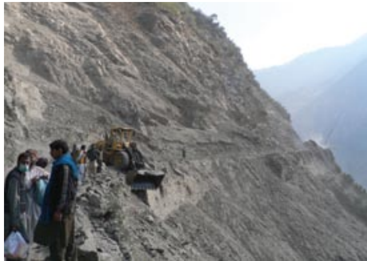
The danger of landslides severely hampered the relief effort until the advice of a slope-stability expert was secured
