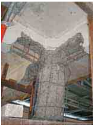
DAMAGED COLUMN, STIRRUPS & ANCHORING ARE NOT ADEQUATE
