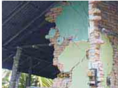
EXAMPLE FAILURE OF WALLS AT THE CORNERS
