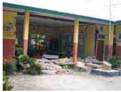
EXAMPLE OF WALL COLLAPSE
