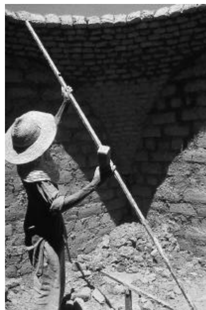
Fig. 8 Using the radial arm in dome building. The arm gives the placement and the angle of every brick.
