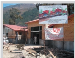
A hospital being built in March 2006 in Balakot, NWFP, claiming to use earthquake resistant materials. Despite the distribution of compensation money to affected families and the introduction of new building codes it is hard to see how they will be implemented in remote areas. Credit: Chris Horwood/IRIN
