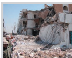
UN HQ at the Canal Hotel (Baghdad) following the 19 August 2003 bomb were senior UN and humanitarian staff were targeted by insurgents opposed to the invasion of Iraq by Coalition forces. The end of perceived neutrality for humanitarians may be part of the 'new aid paradigm'. Credit: UN
