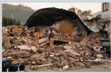
Devastated buildings in the Battagram/Battal area, close to the epicentre of the regional earthquake that was felt as far as Delhi in India and Kabul in Afghanistan. By the final count some weeks later, an estimated 88,000 people fell victim to the quake. Credit: Kamila Hyat/IRIN
