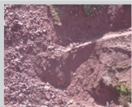
Seven months after the earthquake the access road to Sali Sacha is blocked by new landslides and rockfall. Water and electricity supply is damaged and people struggle to make use of the compensation provided for rebuilding. Credit: Christopher Horwood/IRIN
