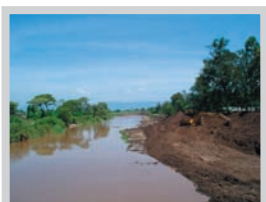
Kenyan government excavator enlarging river beds before the March 2003 rains in Nyanza Province. Credit: IRIN
