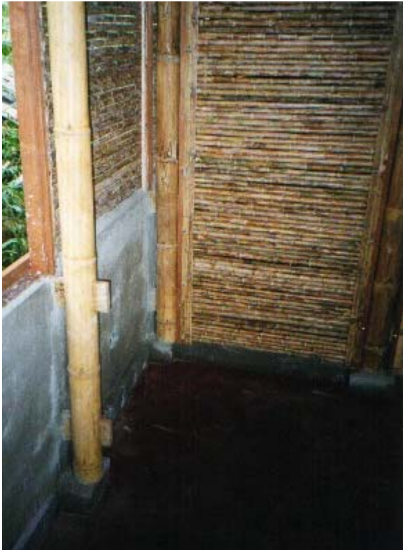
Above: PNB house, detail of unfinished wall. Source: Janssen, personal collection.
