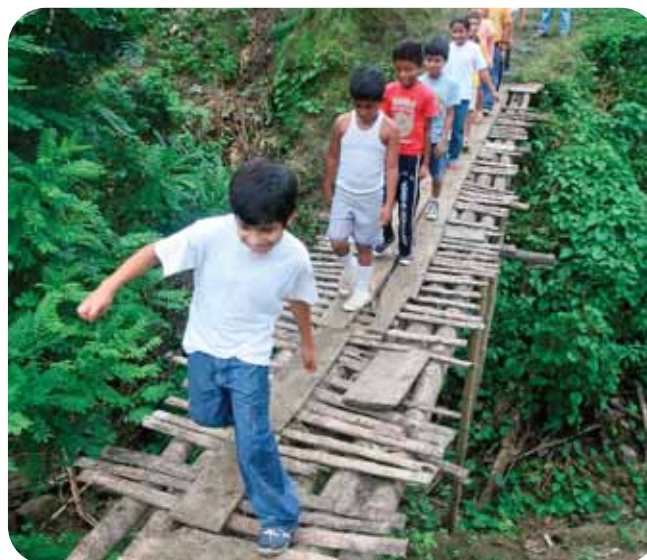
Children in Quebrada de Alajuela, Ecuador, reported the bridge that crosses the village river as posing a safety risk in the event of floods
