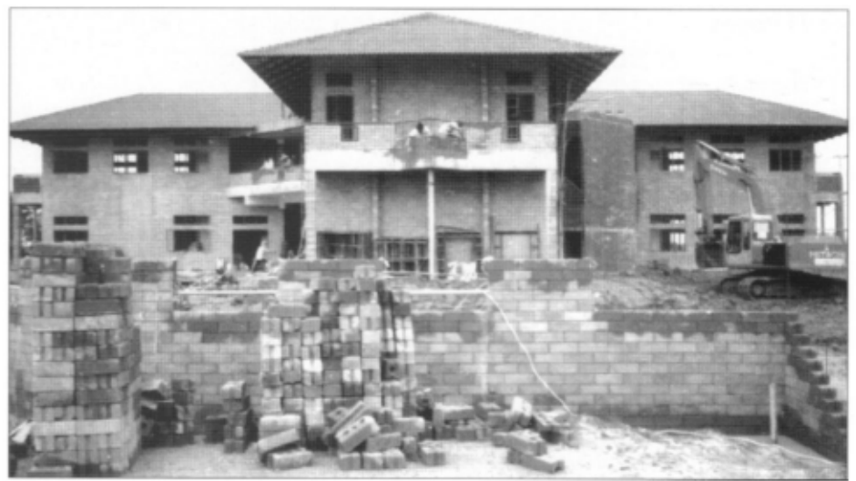
Figure 5 The German School in Chiangmai, Thailand, under construction with load-bearing interlocking concrete block walls
