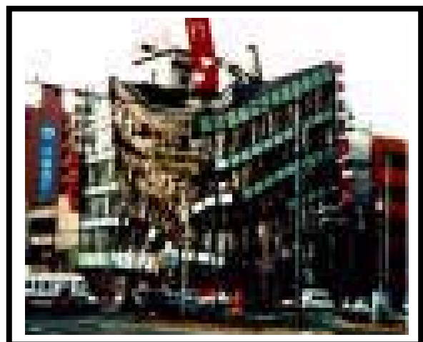
Photo 8 : Effects of the earthquake on reinforced concrete structure
