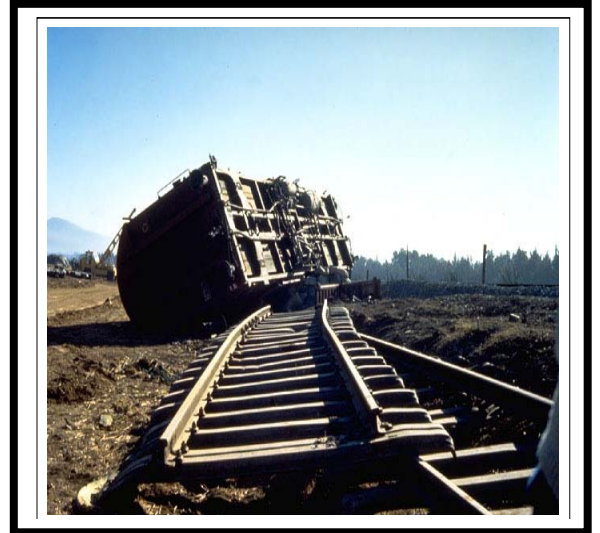
Photo 4: Effect of the earthquake on the rail system during the 2003 Boumerdes earthquake.
