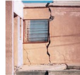
Big vertical crack near the window on south wall
