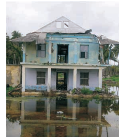
Damage and flooding of the Panchayat building
