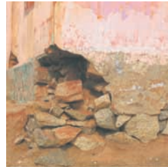
Damage to plinth on south-west corner
