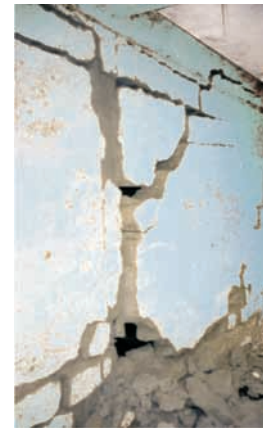
Damage to internal wall of kitchen
