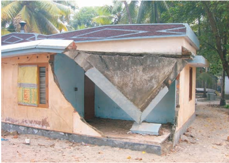
Collapse of north and west walls of the house. Also partial collapse of concrete roof slab
