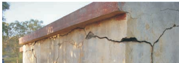
Crack between concrete slab and wall visible on east wall
