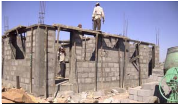
Approximately one million houses were needed to be reconstructed or repaired after the 2001 Gujarat earthquake.
