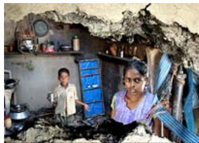
A house in Bihar state severely damaged by the floods in August. AIDMI is covering its beneficiaries with microinsurance against losses to future hazards.
