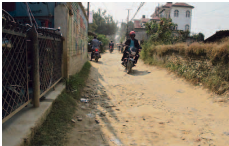
Photo 7o: Damaged black topped inner road in Kathmandu © UN-HABITAT
