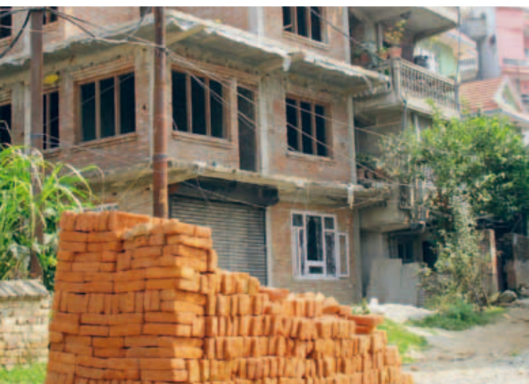
Photo8a: Poor quality bricks © UN-HABITAT
