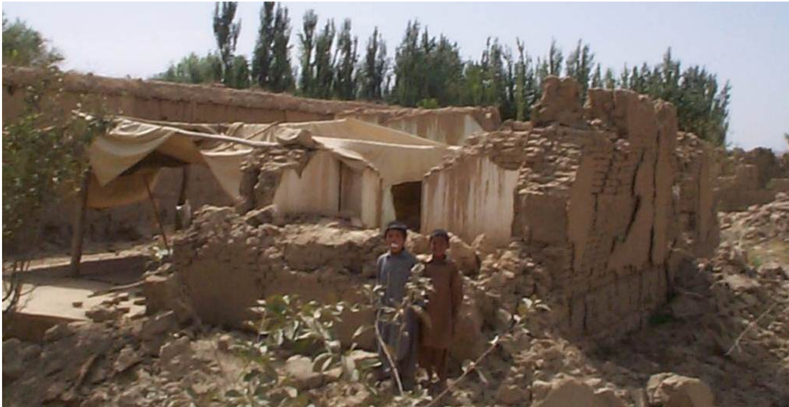
Mix of old and new/compromised practices. The old structure stands but the new ones collapsed
