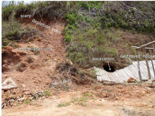
Figure 10: Slope excavated for house building and the consequent small slides above (left) the excavated zone (PK 189 of the RN2)
