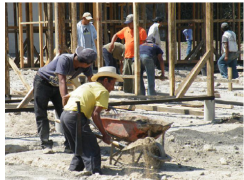
Members of beneficiary families contributed labor to the project in rotating work teams. With technical assistance and construction materials provided by USAID and CRS, the beneficiary families constructed 60 shelters and assisted with the installation of the water and sanitation systems. Julio César Morales/Parish of San Lucas Tolimán
