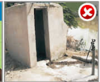
Distance between hand pump and latrine too short.
